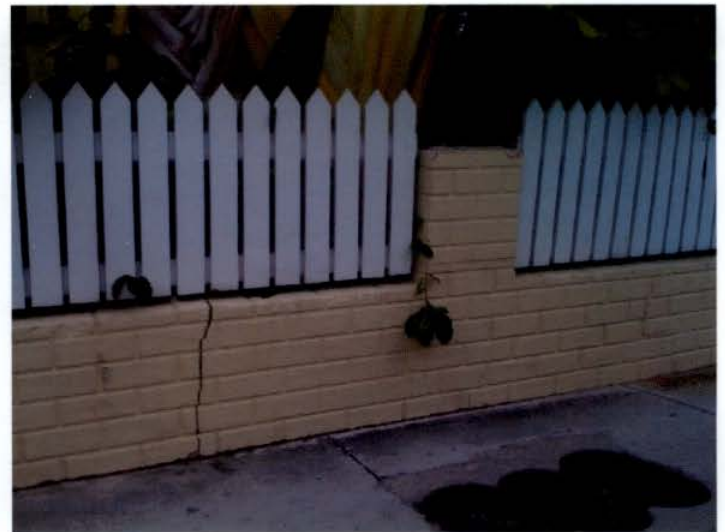
Obvious crack and center stile which has broken off
