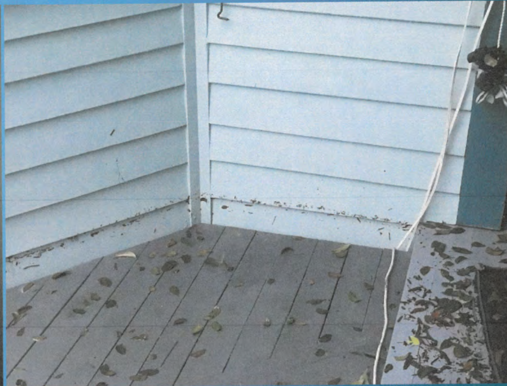
High Water Mark over deck and at interior floor level
