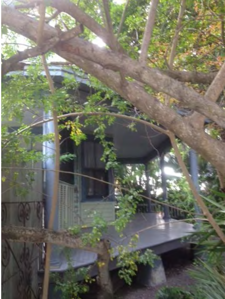
Photograph taken looking south of side of front porch before elevation of house. Tapered concrete footer can be seen in this photograph.
