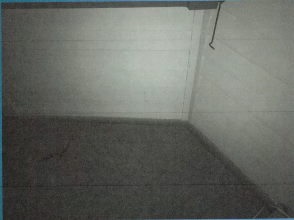
Water Over Deck
