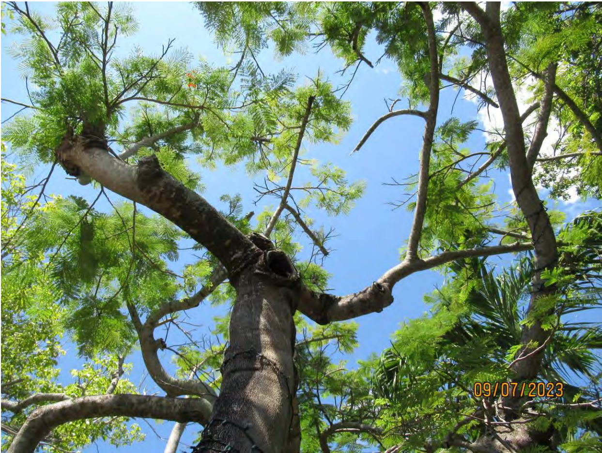
Two close up photos of canopy branches with decay, views 10 & 11.
