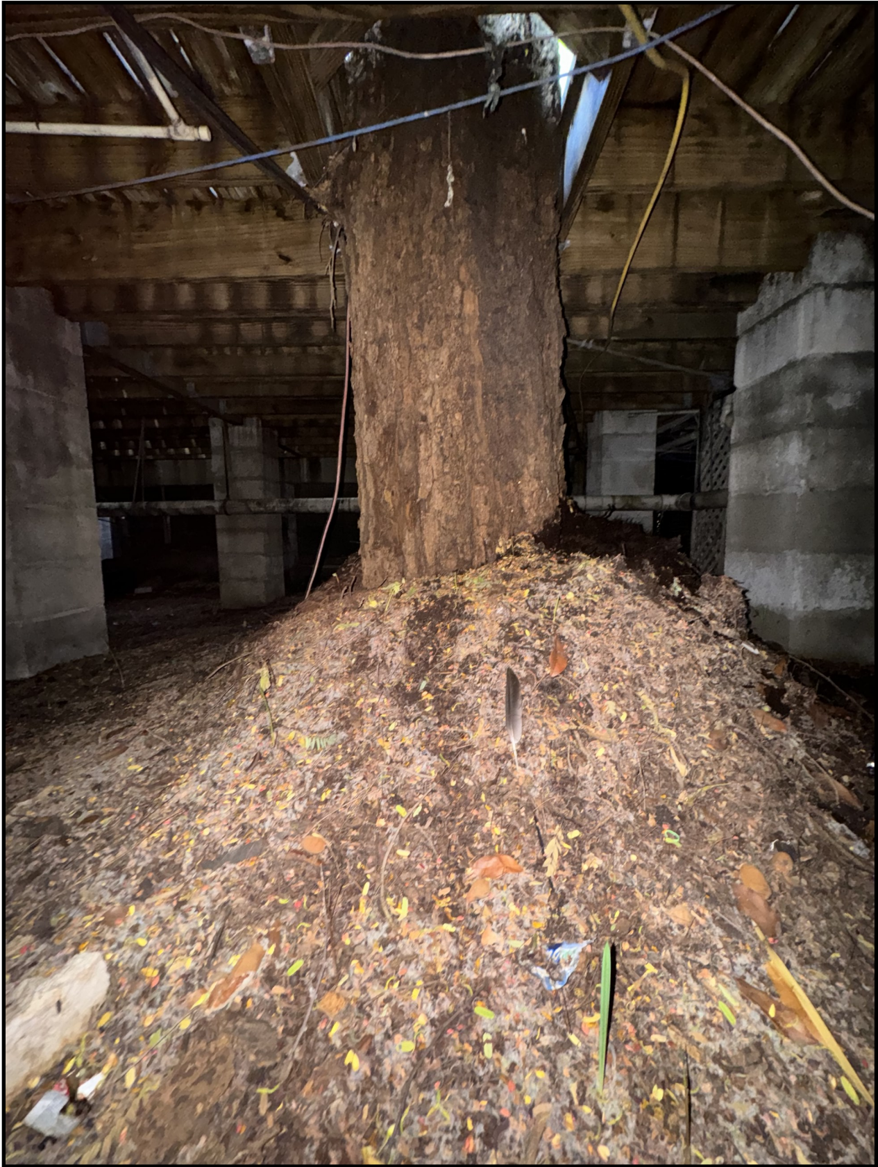
There is over four feet of soil piled around the base of the tree trunk at the ground level, under the decking.
