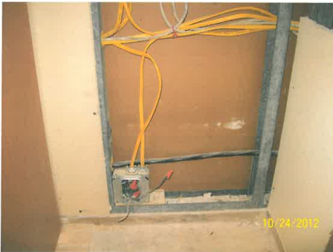
Further electrical installed to accommodate new kitchen appliances. No plumbing or electrical permits on this date.
