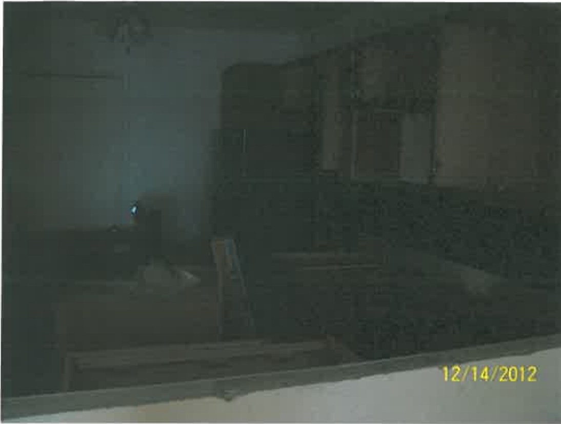
Another angle of the cabinets being removed to access plumbing and electric lines. No electrical or plumbing permits on this date.
