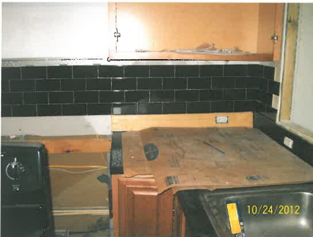
Second Site visit conducted by Inspector Corbett on 24 October 2013 with Key West by the Sea Property Manager and Plumbing Inspector Wayne Giordano to confirm that work had been done after the stop work order was issued. Cabinets were installed to the wall, further electrical outlets installed and a tile backsplash has been installed. No plumbing or electrical permits on this date.
