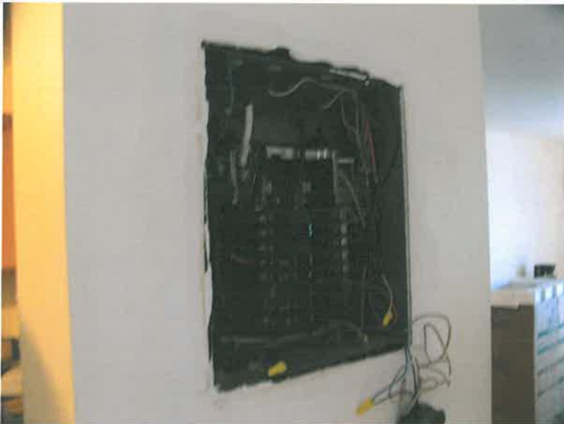
Work being performed by Mr. Roloff on 2 October 2013 Photo taken by Inspector D Ray Electric box has been altered.
