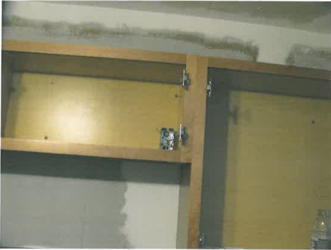
Work being performed by Mr. Roloff on 2 October 2013 Photo taken by Inspector D Ray. Cabinet backing installed to a newly installed drywall with wet paste.
