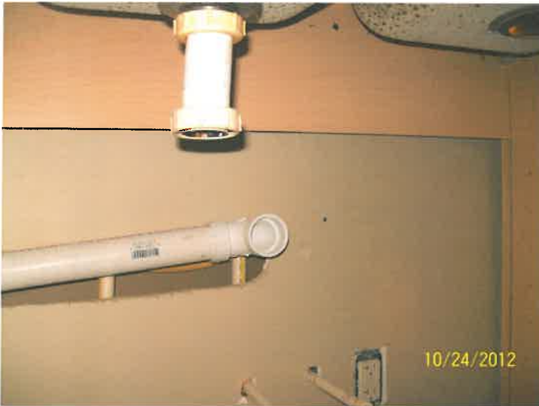
Open plumbing line. New electric socket installed. No permits for plumbing or electric on this date.
