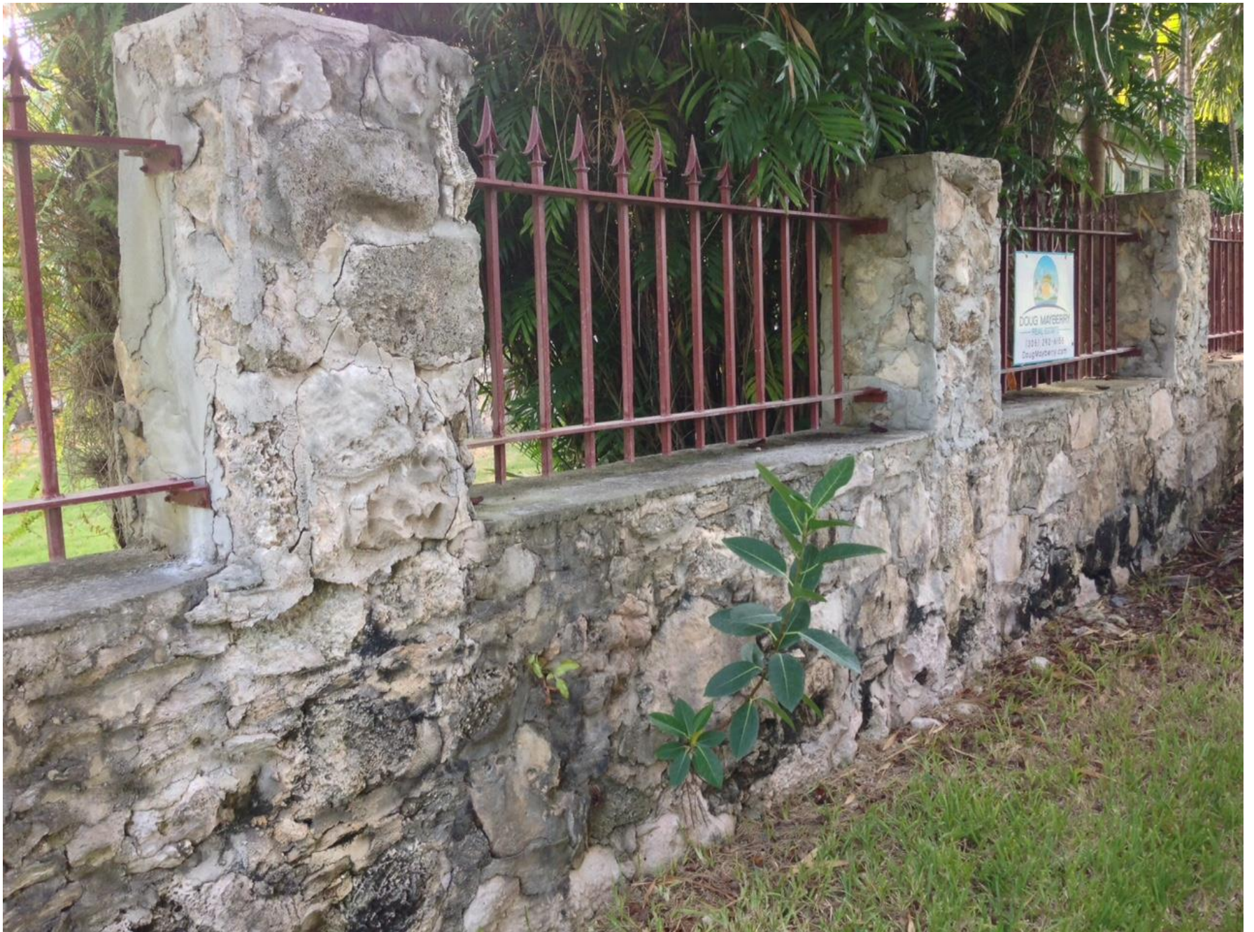
The center portion of this wall to be demolished for pedestrian access.
