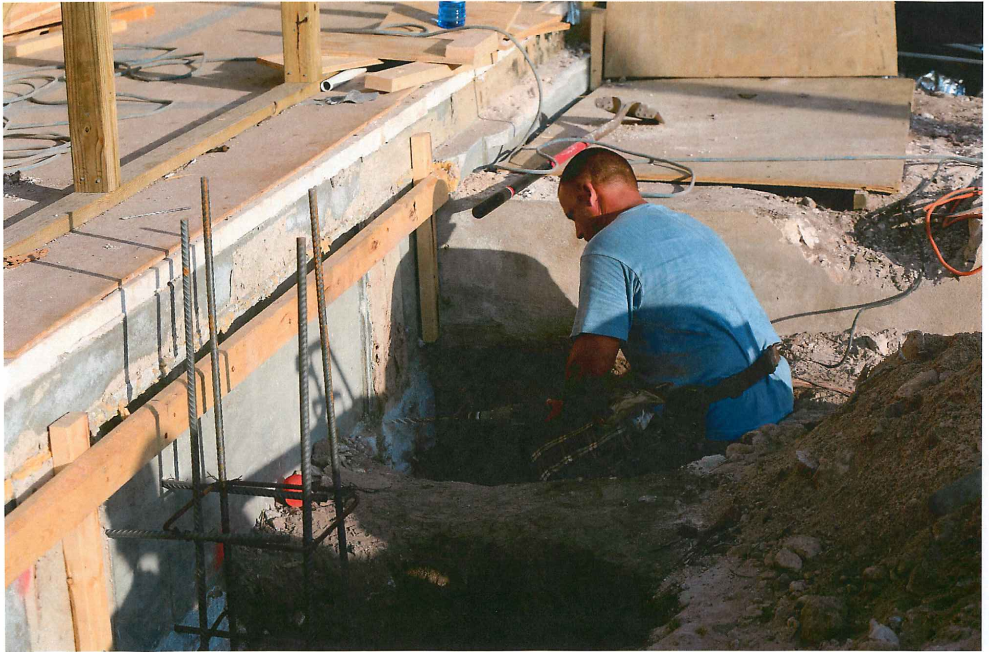
New foundation piers to carry increased loads old foundation piers were set on top soil
