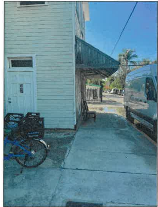
Image depicts the side view of the historic structure and wooden overhang.
