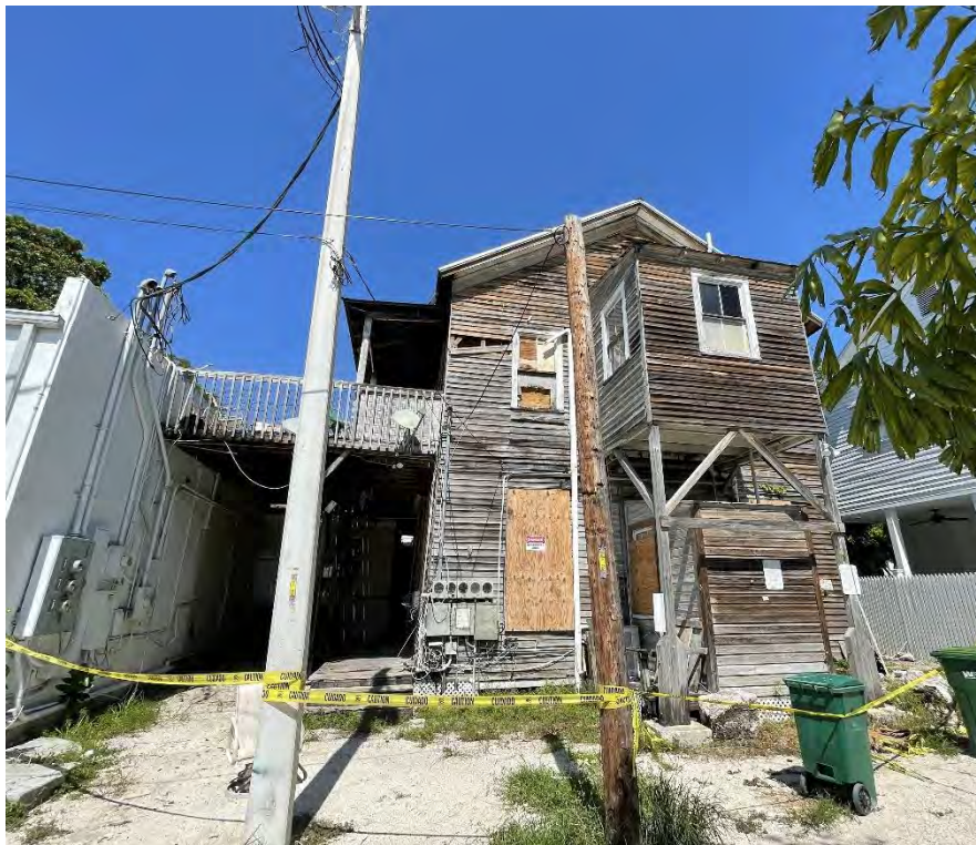
Front elevation after the fire.
