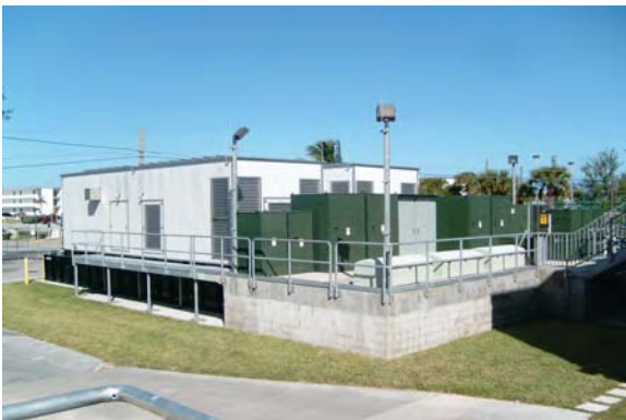
JIATF South, Emergency Generators (1.5 MW)
