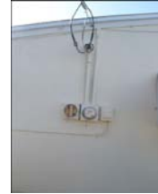
Old meter center. Can be raised, but needs meterpack
