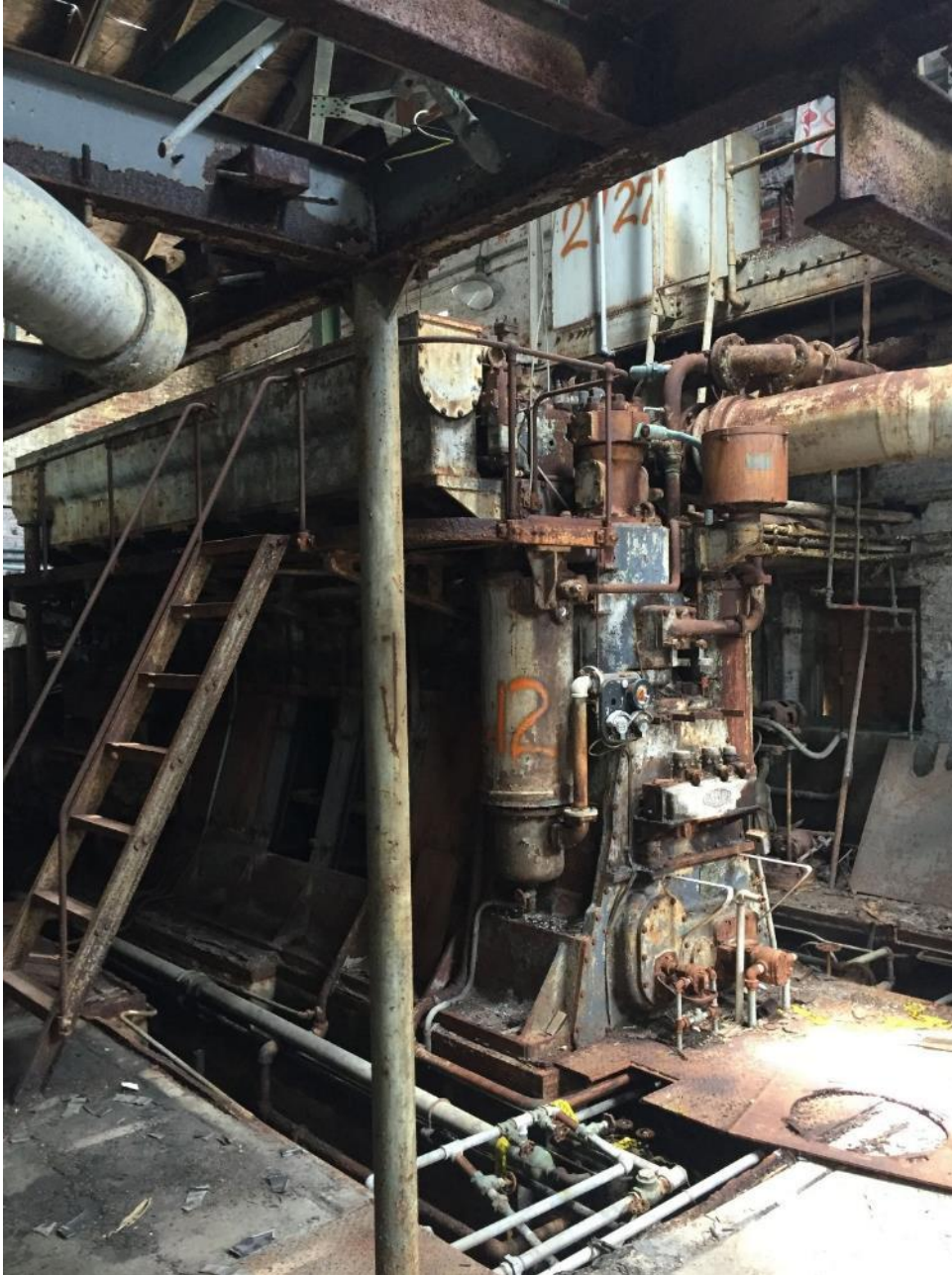
PHOTO 2: Inactive generator inside buildings at the Site
