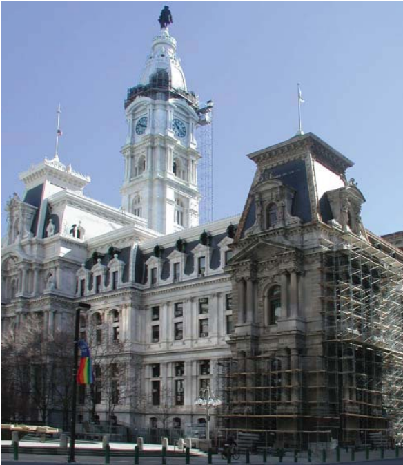
The building during restoration- left side shows newly cleaned stone while the right side awaits cleaning
