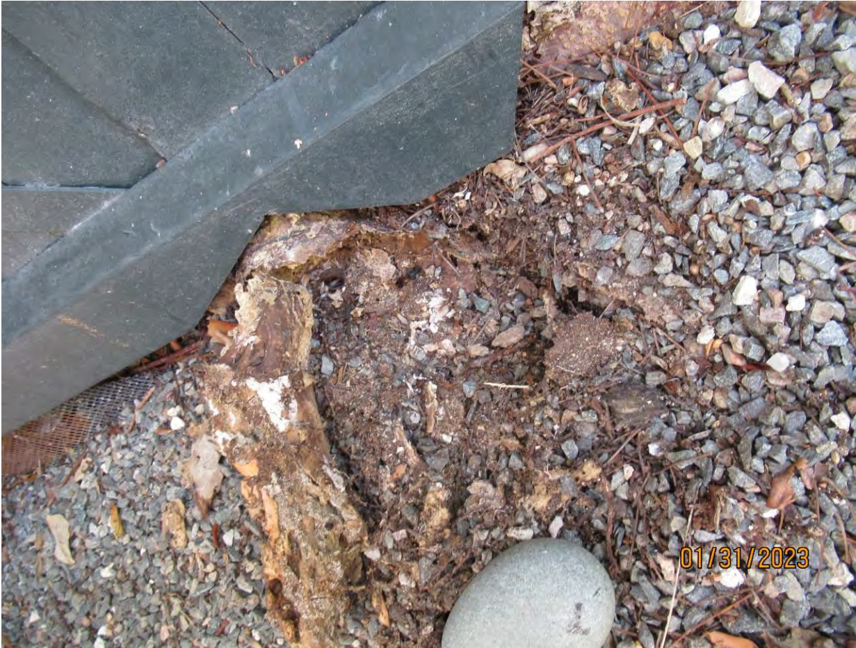
Photo of decayed root area on 915 side of tree showing nest of carpenter ants.
