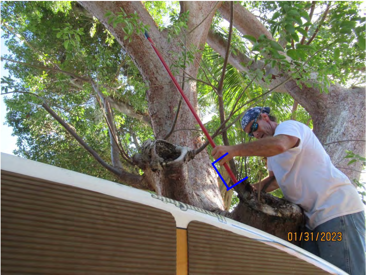
Photo showing length of stick that penetrated the decay of cut area 1 (approx. 6-8 inches).
