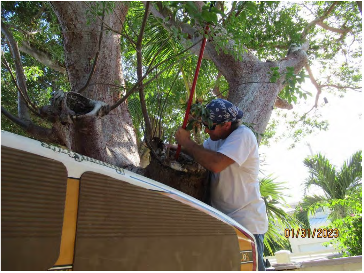
Photo showing measuring stick in decay area 2.
