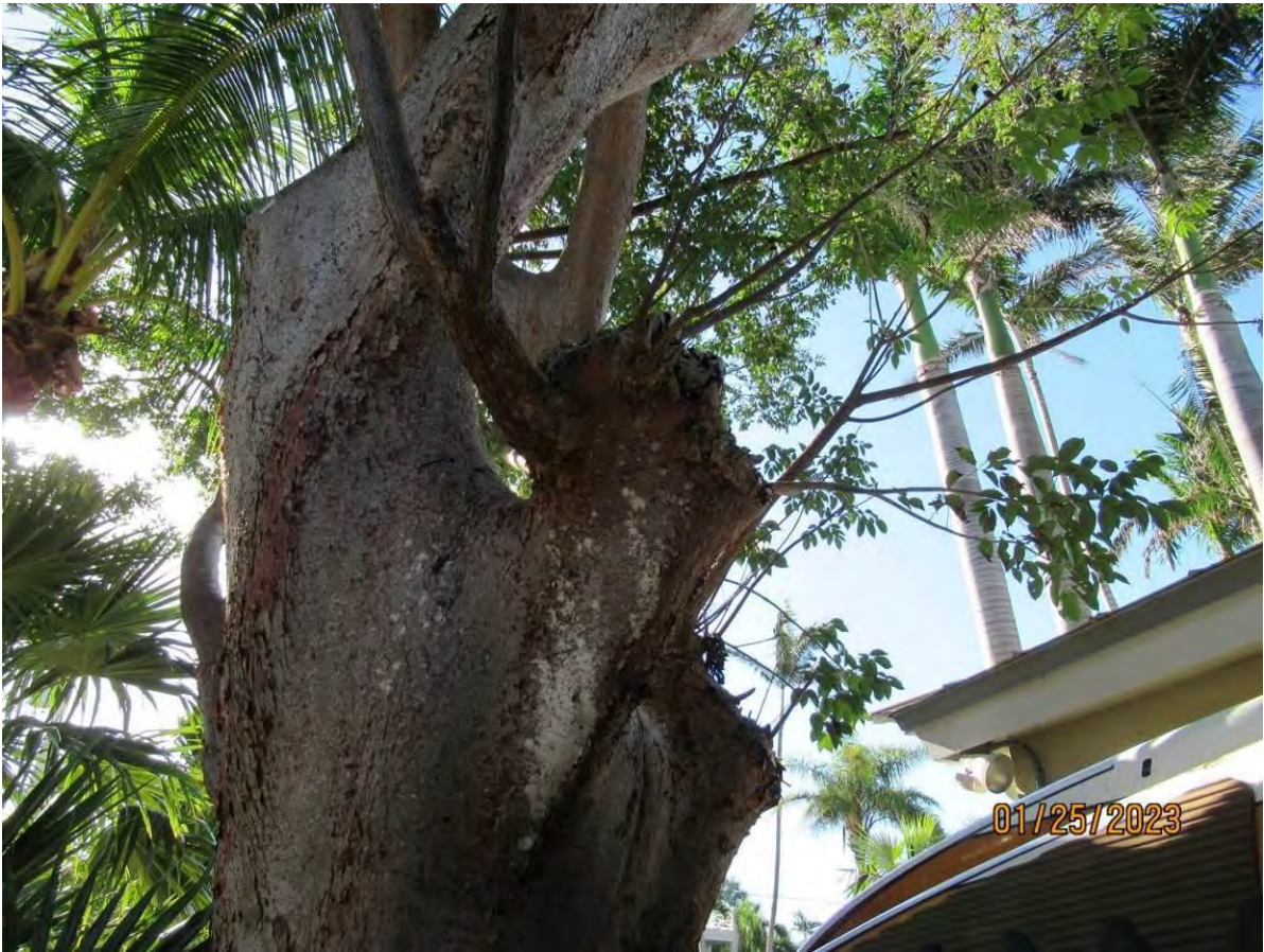
Photo of old cut decay areas 1 and 2 from 923.
