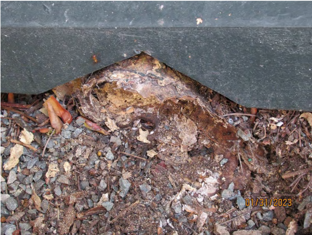
Close up photo of decayed root area on 915 side of tree.
