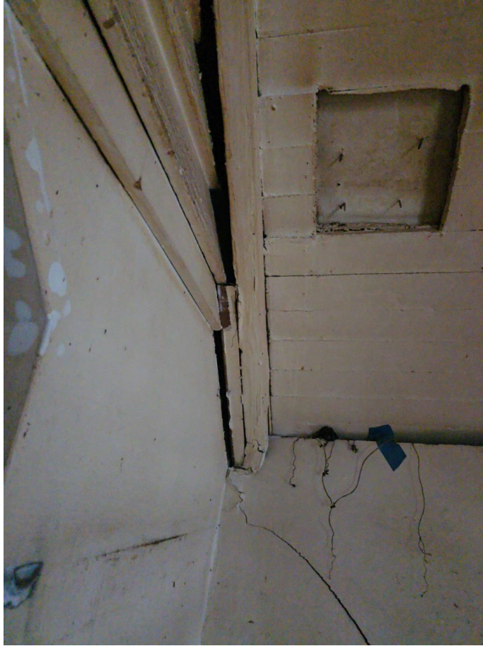
SEPARATED ROOF FRAMING
