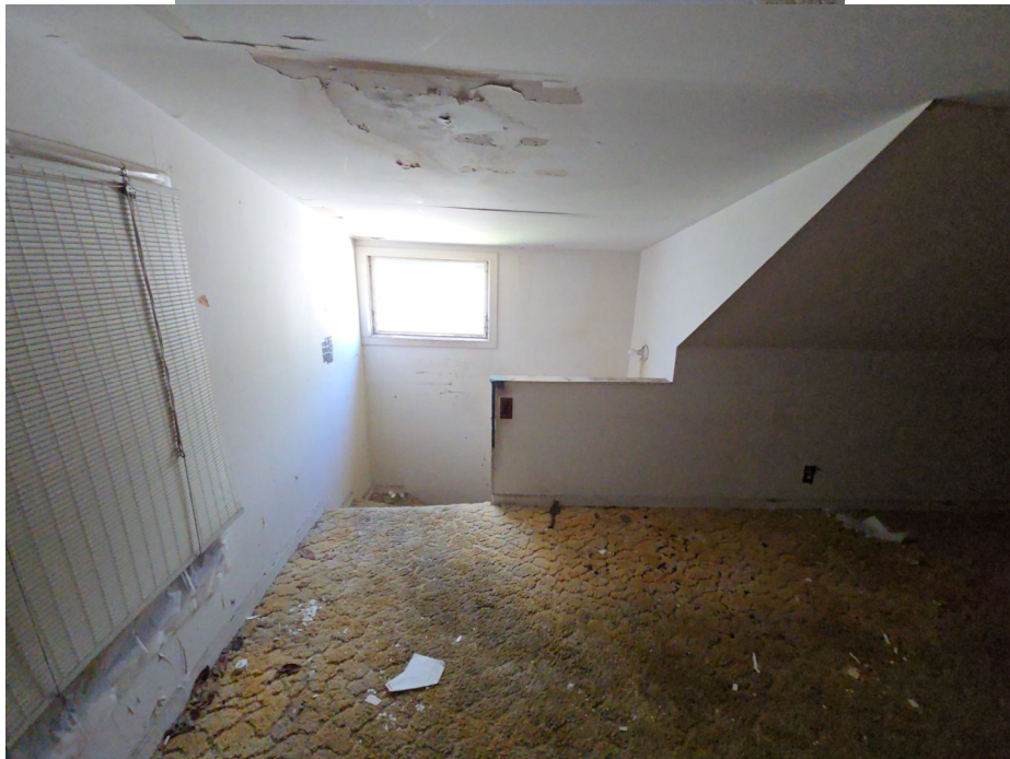
1/2 STORY WATER DAMAGE
