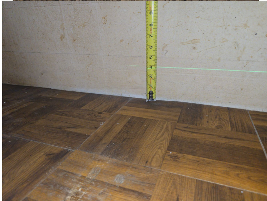
UNLEVEL FLOOR (SUNKEN FOUNDATION & FRAMING)
