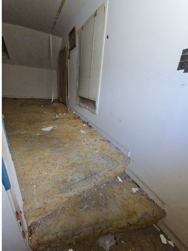
1/2 STORY WATER DAMAGE
