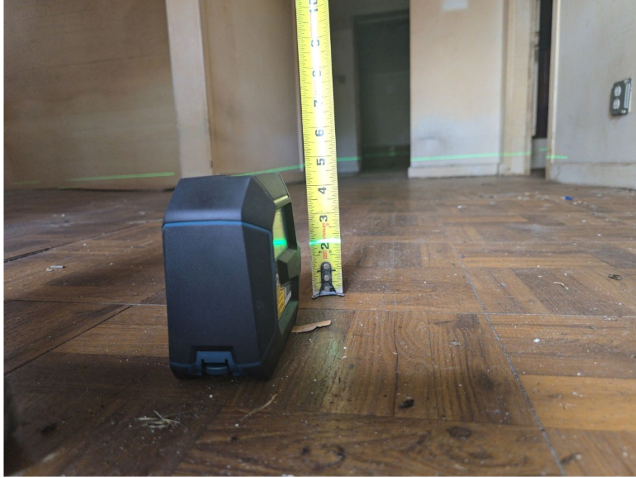
UNLEVEL FLOOR (SUNKEN FOUNDATION & FRAMING)
