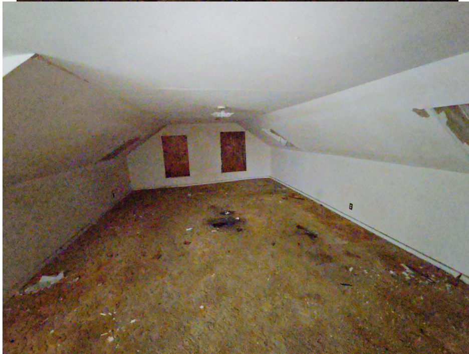
1/2 STORY WATER DAMAGE
