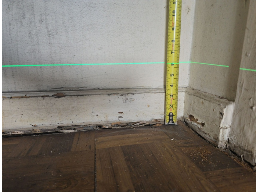
UNLEVEL FLOOR (SUNKEN FOUNDATION & FRAMING)
