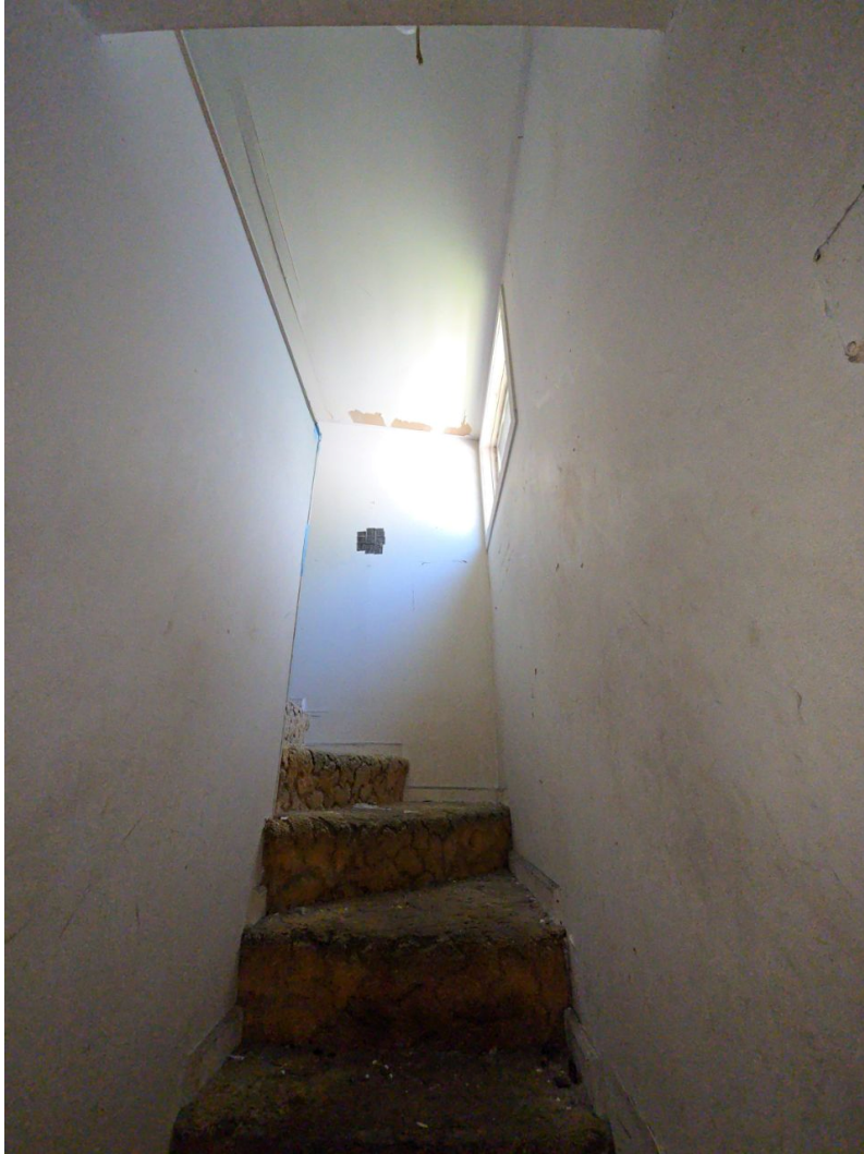
½ STORY WATER DAMAGE
