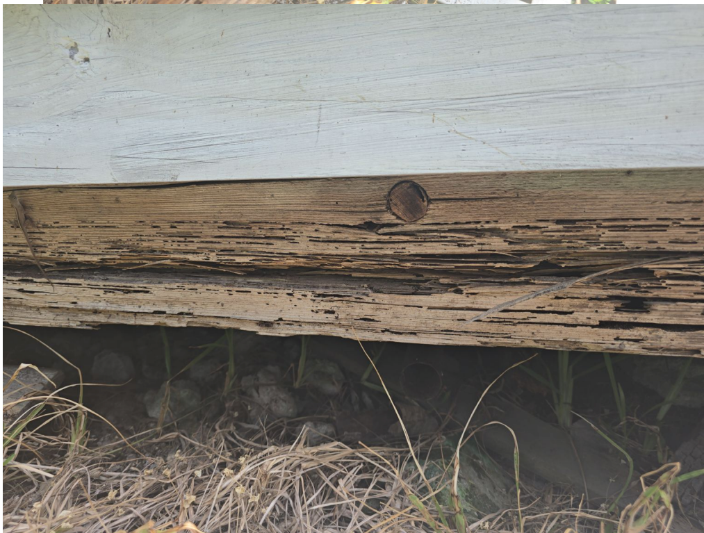
DETERIORATED RIM JOIST
