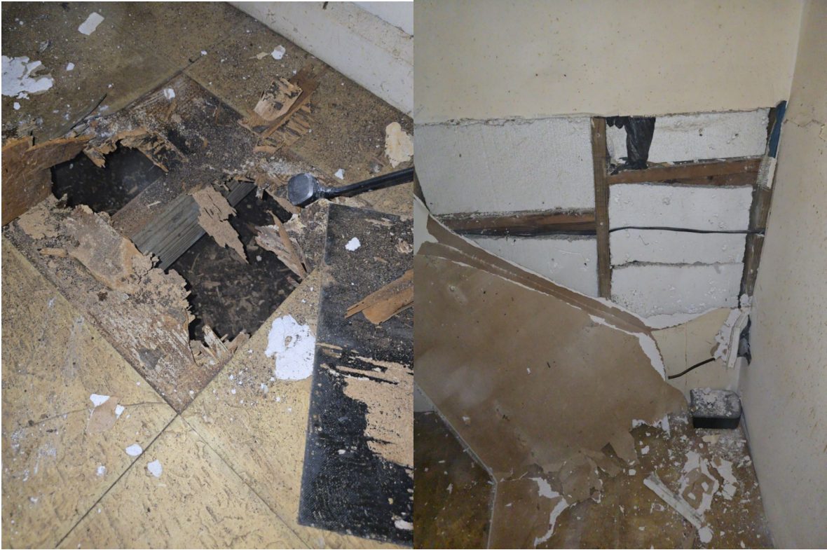
DETERIORATED FLOOR FRAMING & SHEATHING
