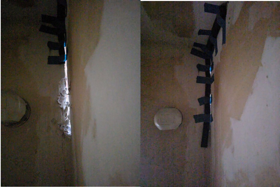
DETERIORATED WALL CONDITION (SEPARATION)
