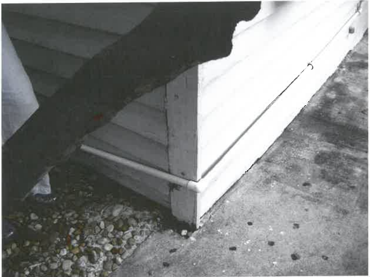
More wood rot and piping not supported
