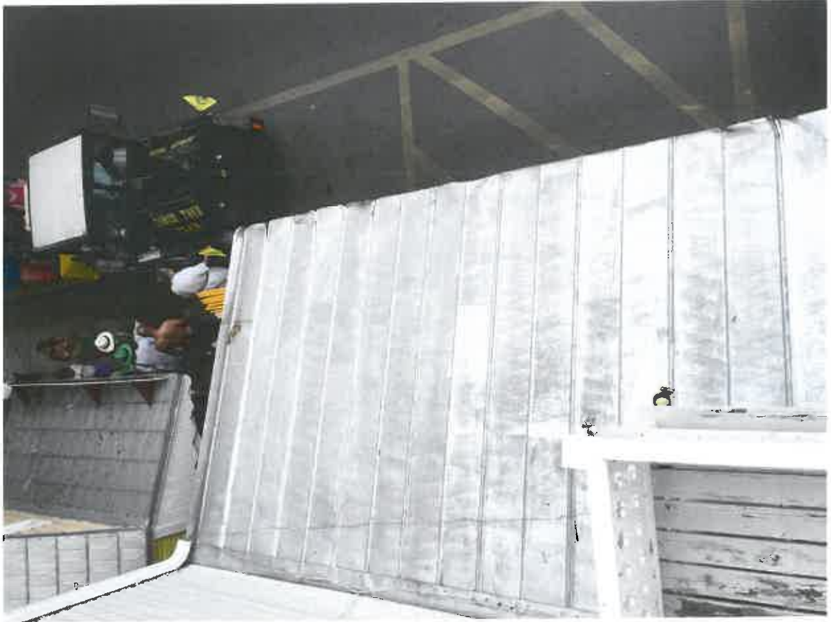
Lower roof damaged by trucks
