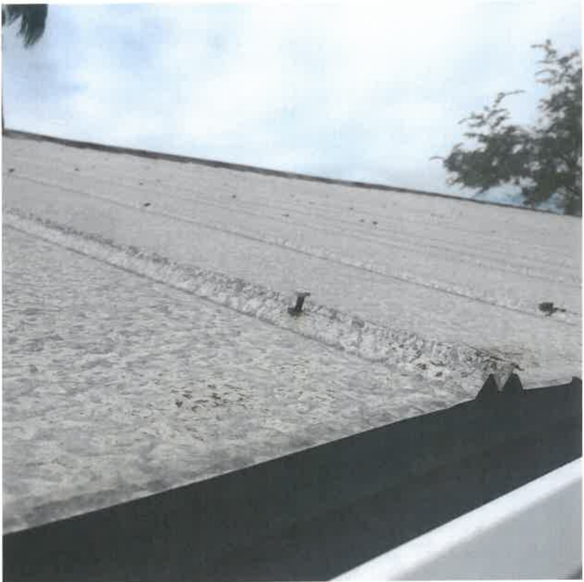
Roofing nails pulling loose
