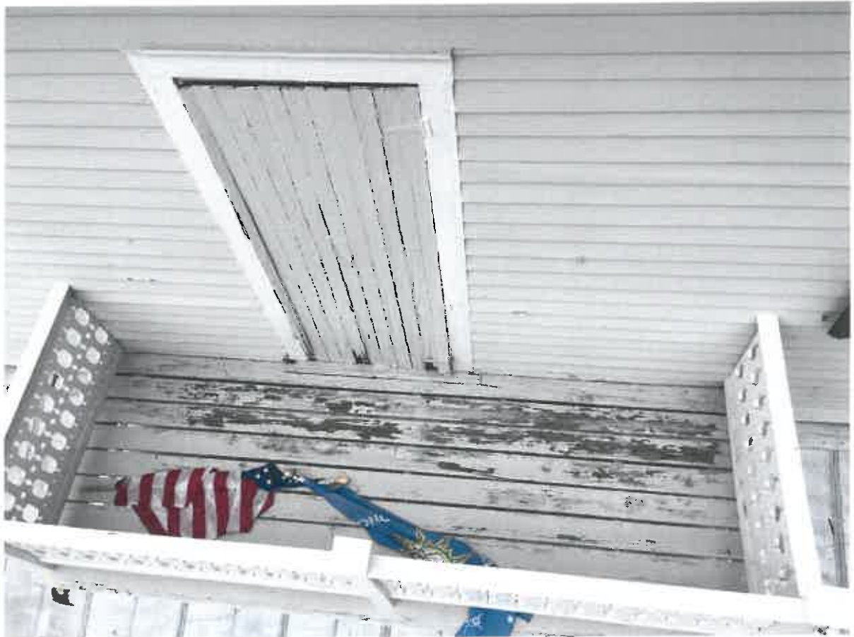
Porch loose and in need of repair
