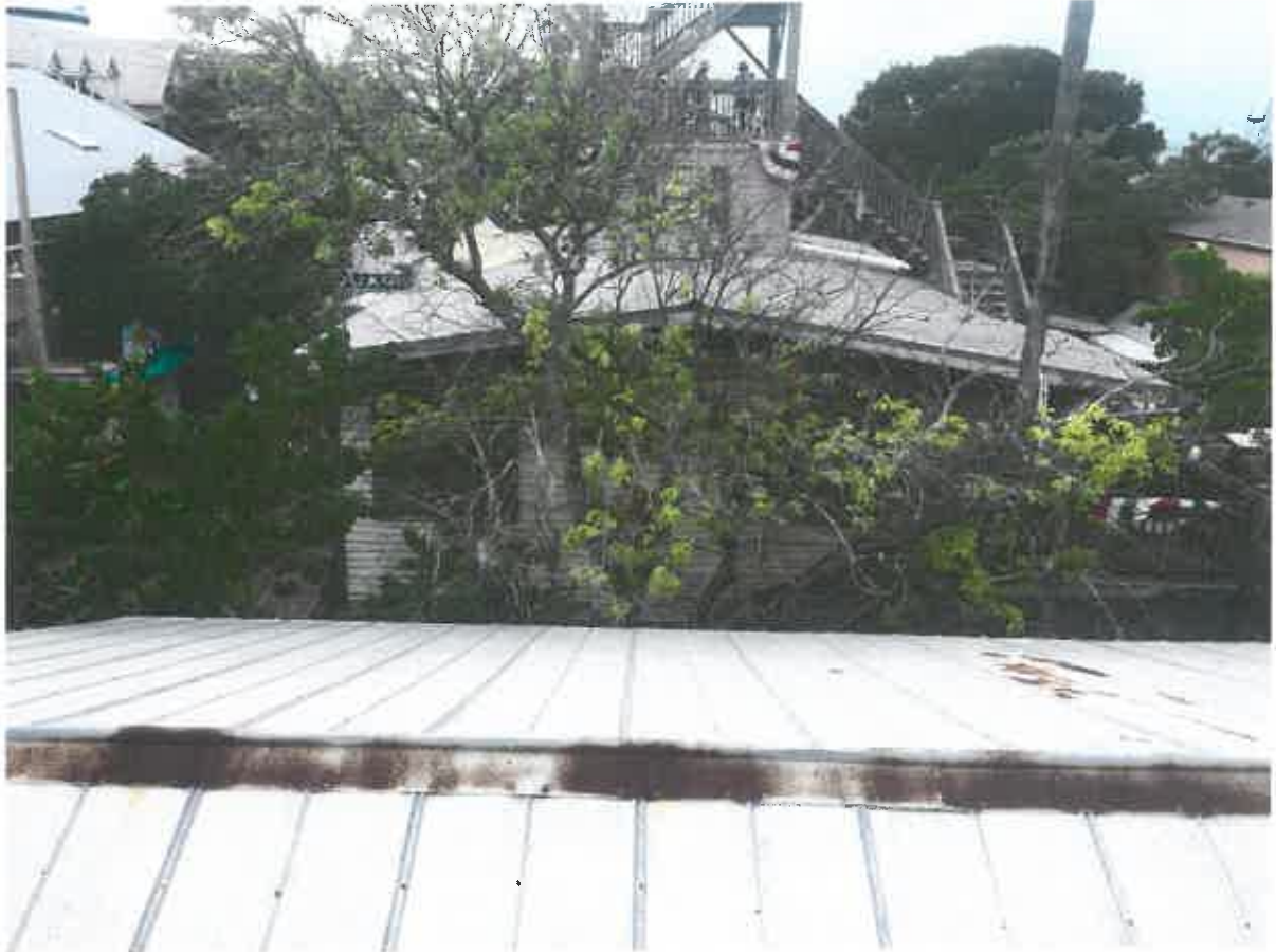
Roof damaged by trees
