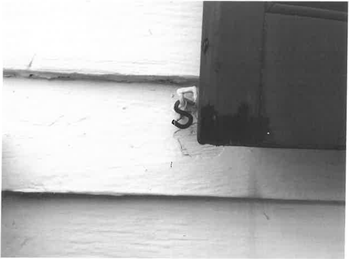
Shutter needs replacing
