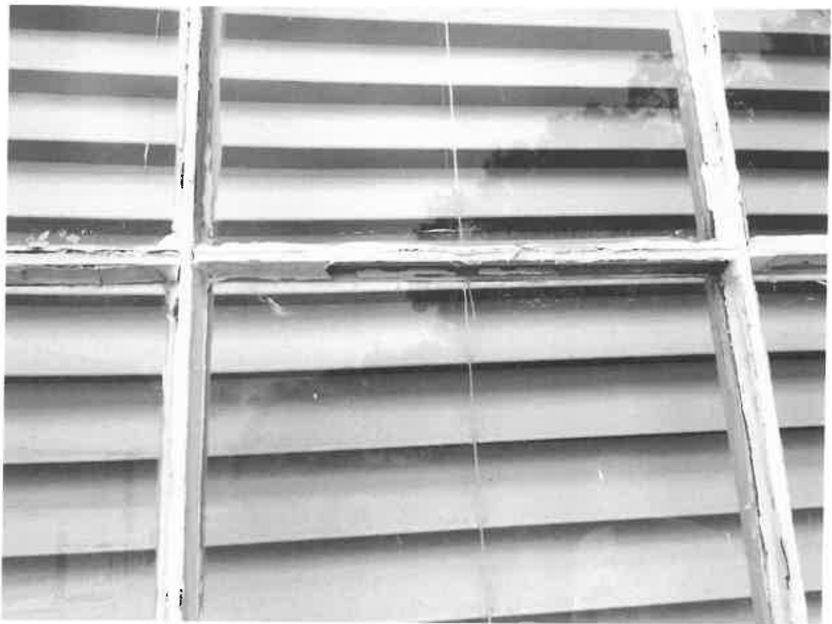
Outside window glazing bad
