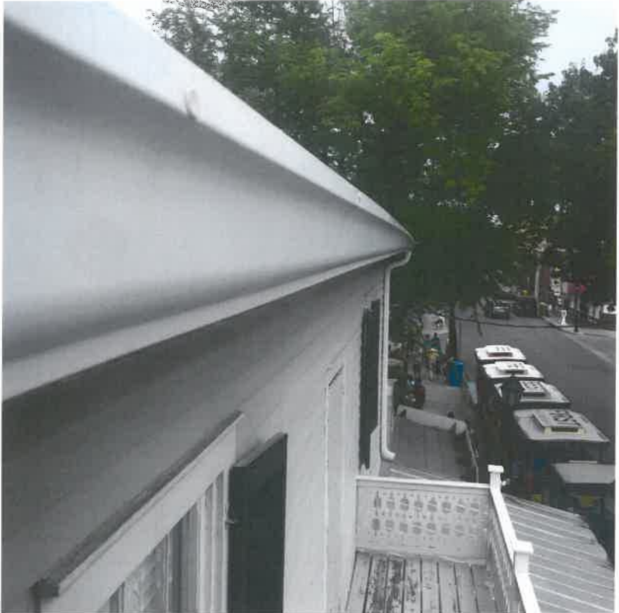
Gutter has sags and the run is holding water
