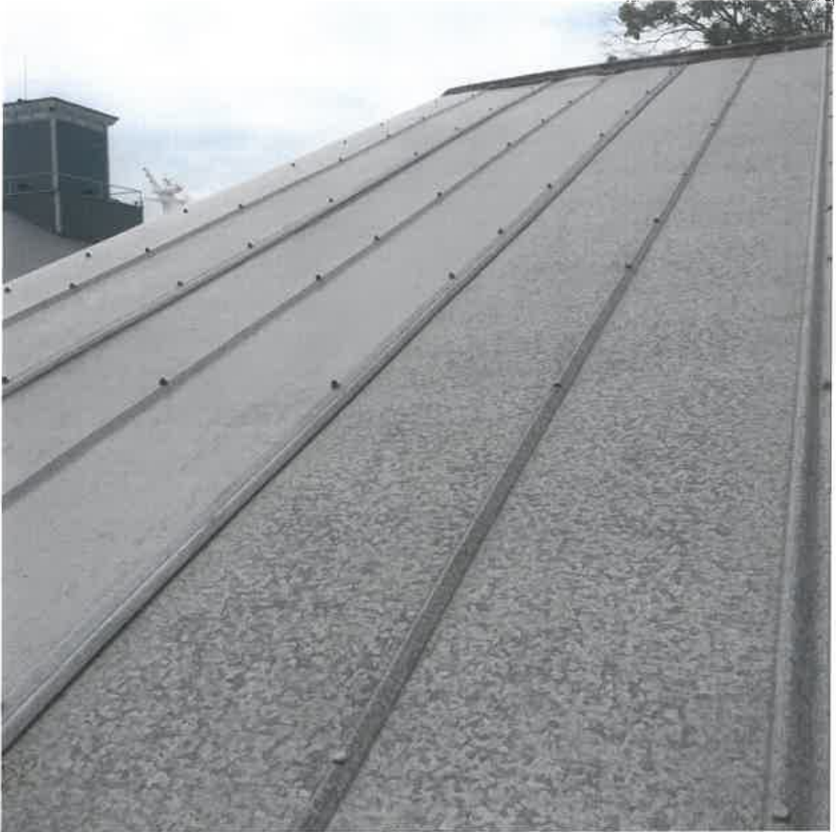
Old roofing needs replacing
