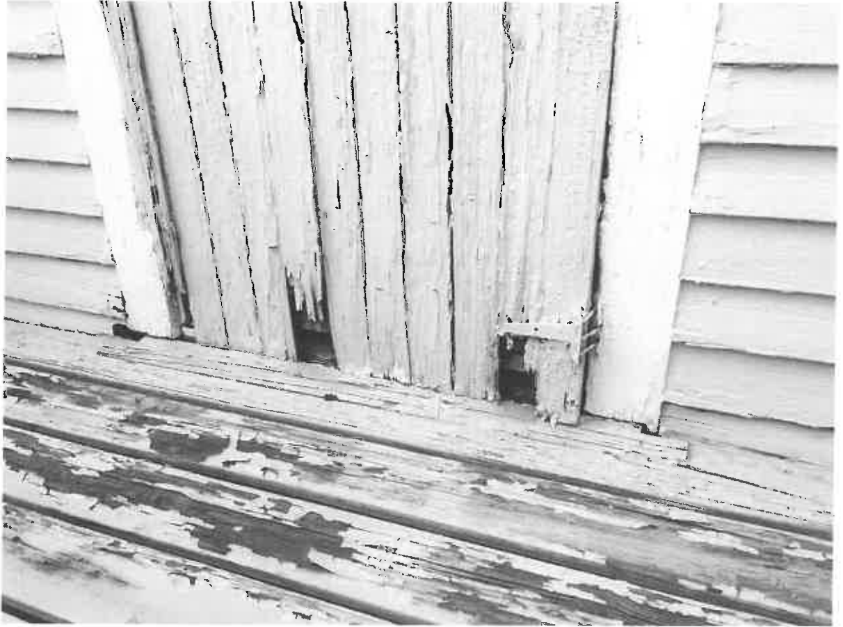
Outside door needs to be replaced
