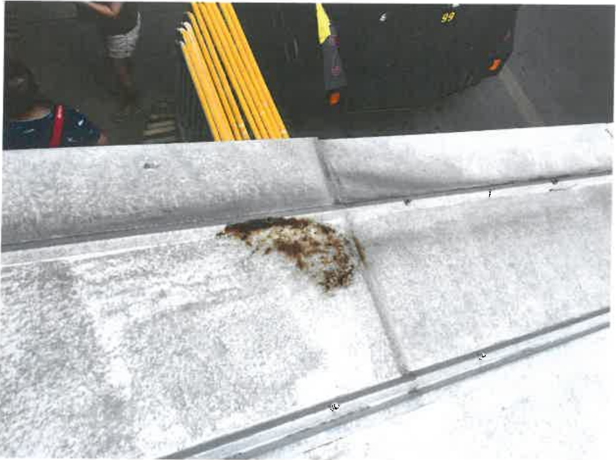
Roof rusting and roof gutter draining on lower roof
