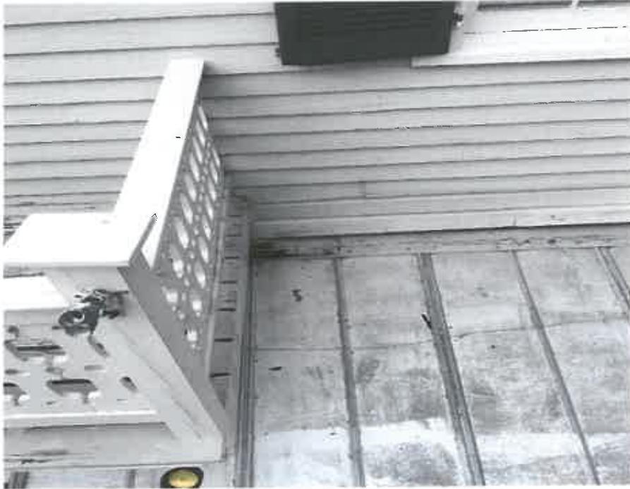
Flashing rusting. Needs repair
