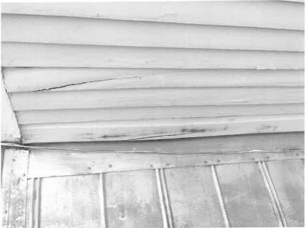
Second floor siding splitting and cable unsecured
