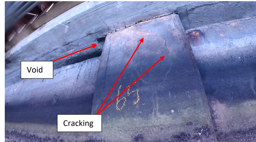
Deficiency B-69: Pile/Cap 107 (Station 7+71)
