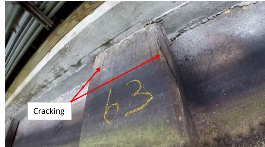
Deficiency B-67: Pile 105 (Station 7+55)
