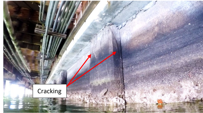
Deficiency B-60: Pile 97 (Station 6+90)
