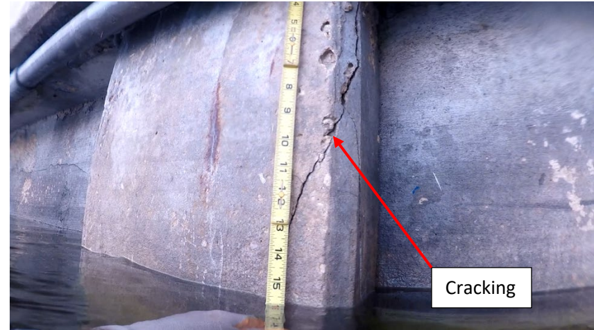
Deficiency A-13: Pile 18 (Station 1+47)
