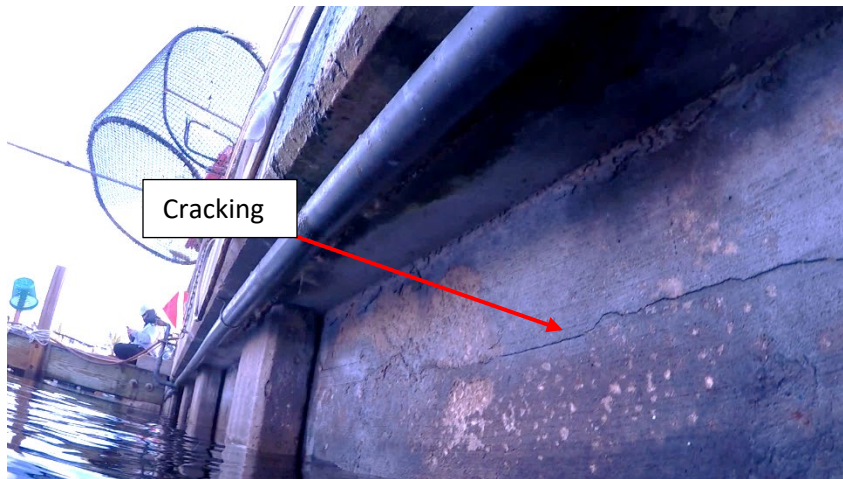
Deficiency A-14: Panel 18-19 (Station 1+50)
