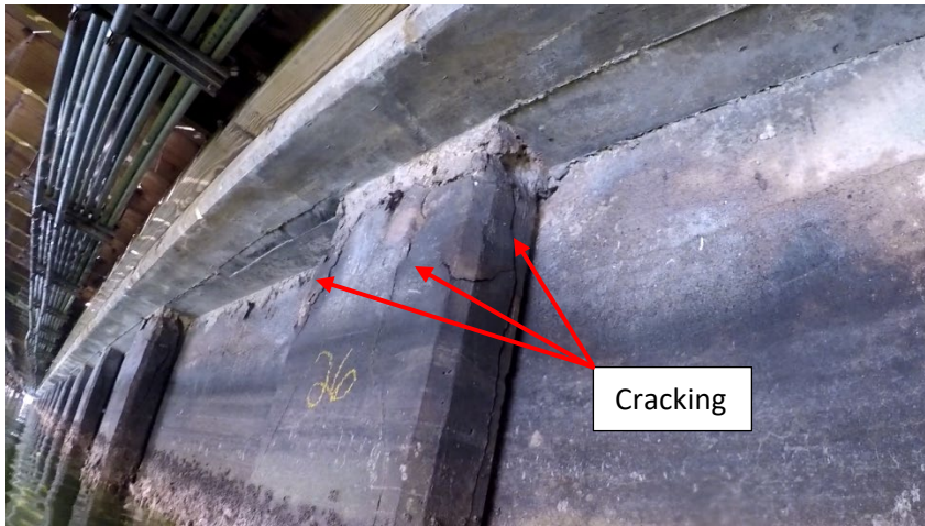
Deficiency B-47: Pile 68 (Station 4+63)
