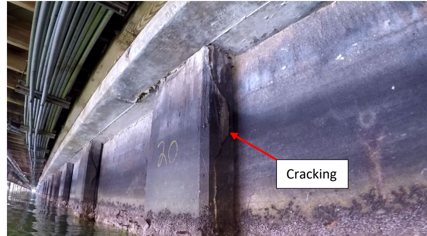
Deficiency B-42: Pile 62 (Station 4+25)
