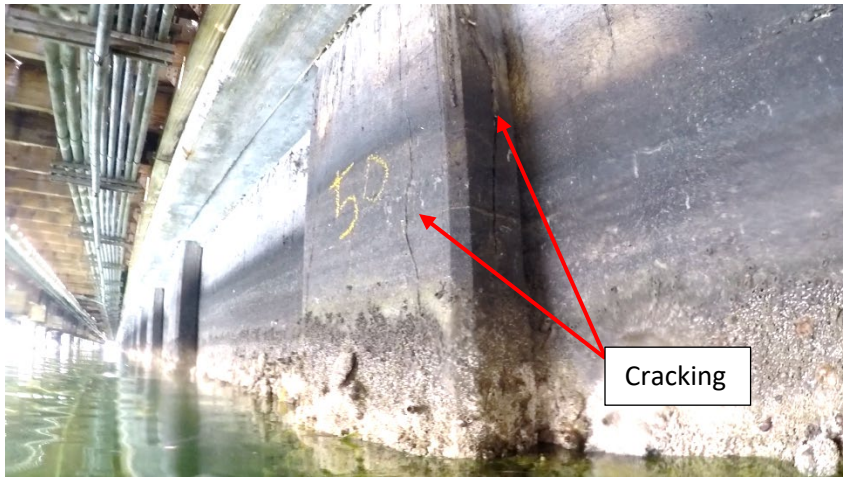
Deficiency B-57: Pile 92 (Station 6+51)
