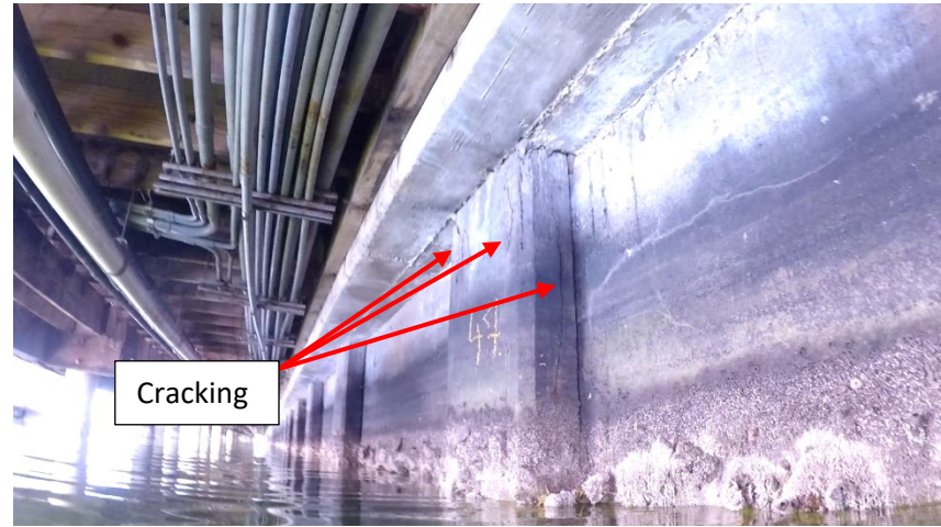
Deficiency B-56: Pile 89 (Station 6+27)
