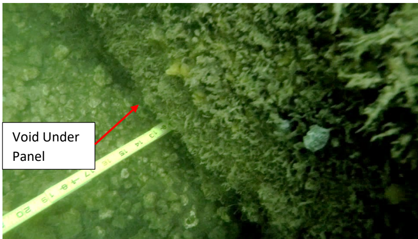
Deficiency A-8: Panel 12-13 (Station 0+75)
