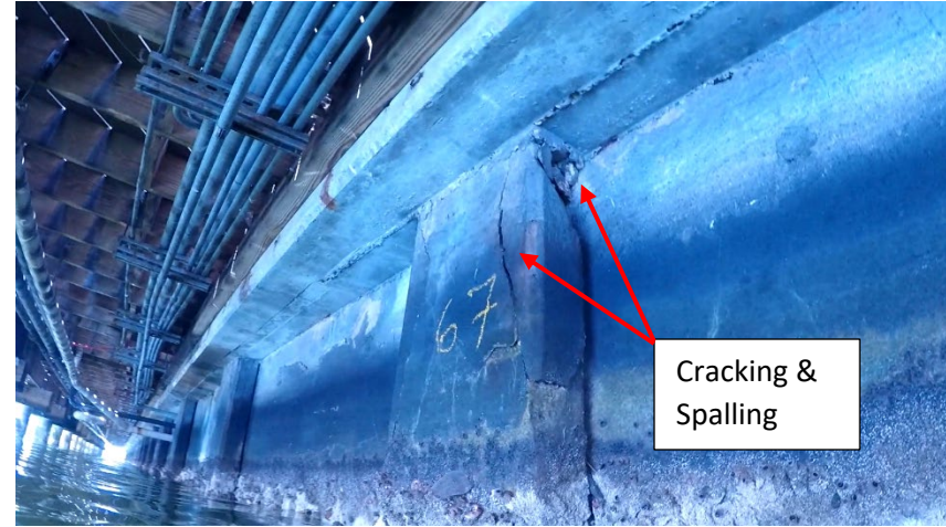
Deficiency B-71: Pile 109 (Station 7+88)
