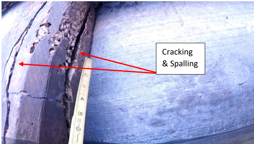
Deficiency A-16: Pile 23 (Station 1+80)
