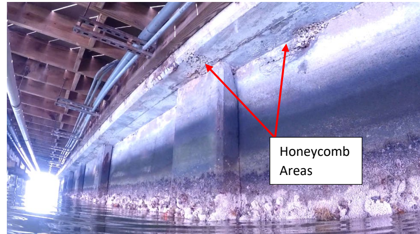
Deficiency B-83: Cap @124-127 (Station 9+04 to 9+25)_1 of 2
