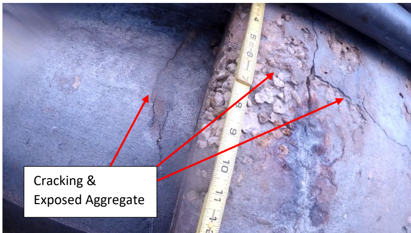
Deficiency A-18: Pile 26 (Station 2+00)_2 of 2
