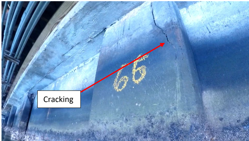
Deficiency B-70: Pile 108 (Station 7+80)
