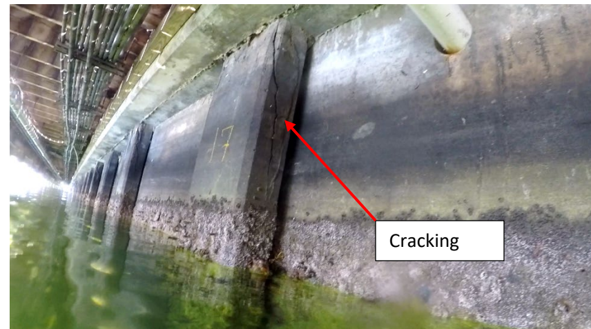
Deficiency B-40: Pile 59 (Station 4+05)
