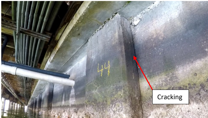
Deficiency B-55: Pile 86 (Station 6+02)
