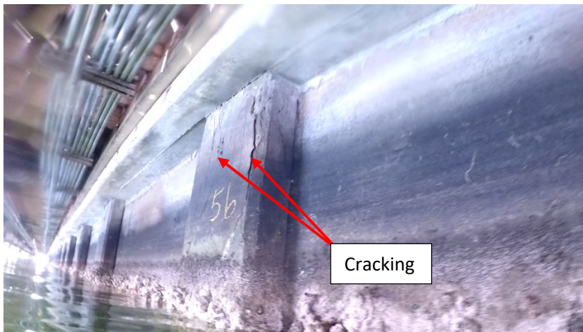
Deficiency B-61: Pile 98 (Station 6+99)
