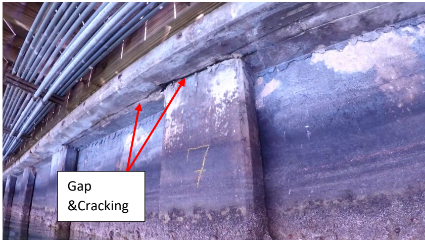
Deficiency B-32: Pile/Cap 49 (Station 3+43)
