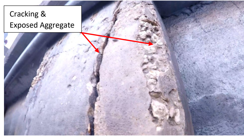
Deficiency A-18: Pile 26 (Station 2+00)_1 of 2
