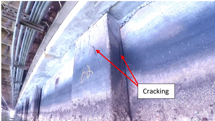
Deficiency B-66: Pile 104 (Station 7+47)
