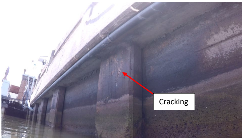
Deficiency B-25: Pile 38 (Station 2+70)
