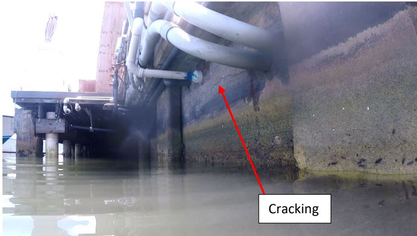
Deficiency B-27: Panel 41-42 (Station 2+93)
