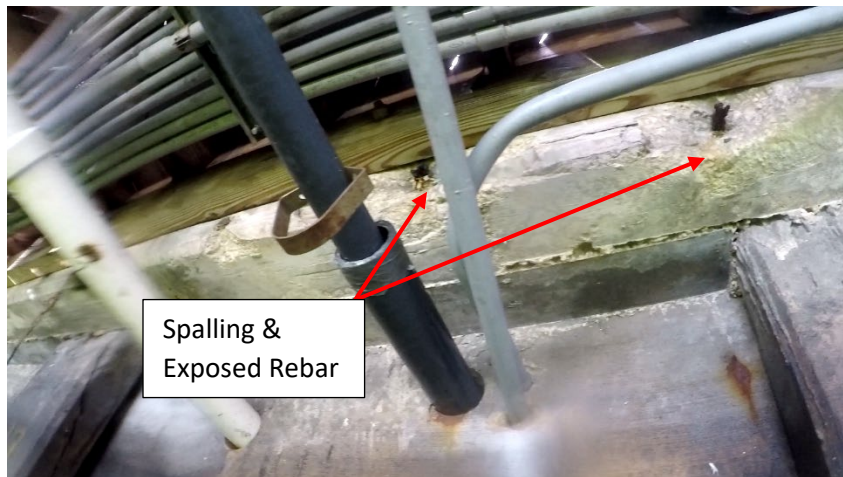
Deficiency B-39: Cap @58-59 (Station 4+01)
