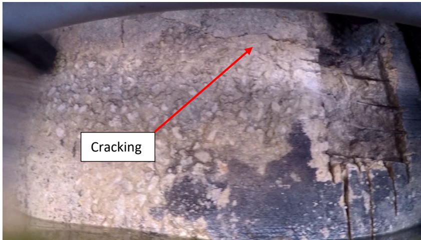
Deficiency A-1: Panel 3-4 (Station 0+14)
