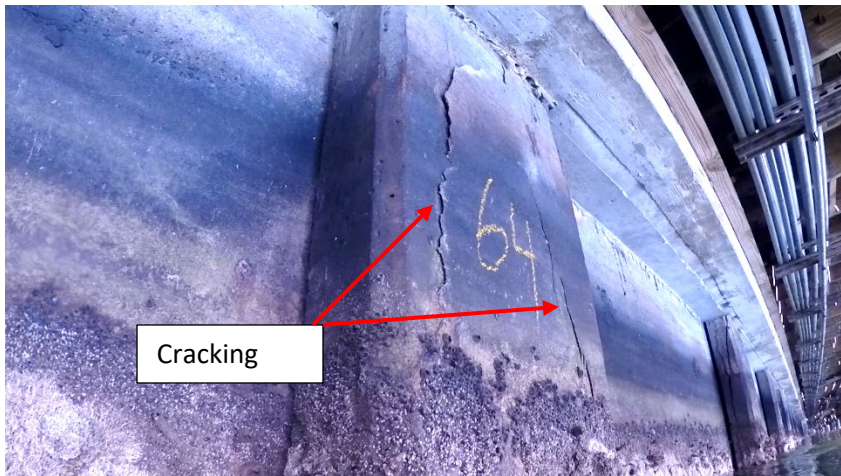
Deficiency B-68: Pile 106 (Station 7+63)
