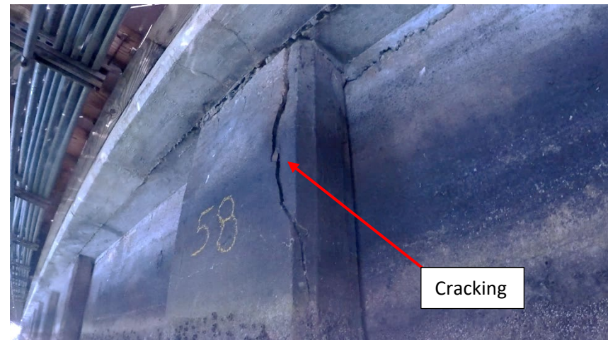
Deficiency B-62: Pile 100 (Station 7+15)
