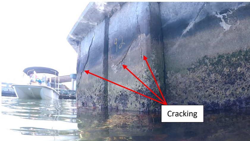
Deficiency B-96/97: Pile 135/136 (Station 9+83/9+86)
