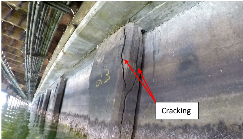
Deficiency B-45: Pile 65 (Station 4+44)_1 of 3
