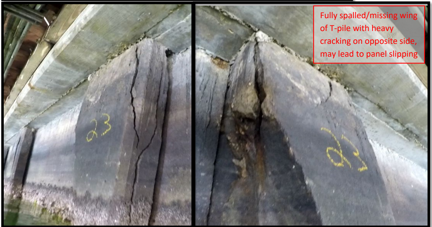
Figure 10: Critical Deficiencies – [Top] A-4 (Station 0+39), [Bottom] B-45 (Station 4+44)
