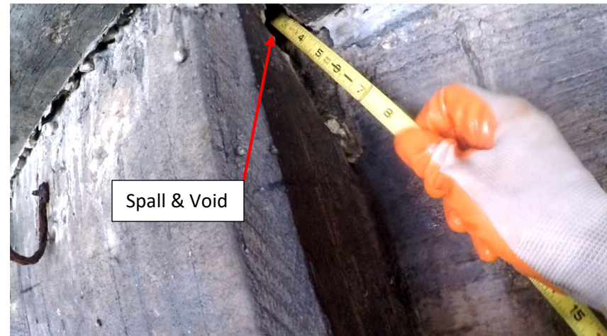
Deficiency B-52: Pile 73 (Station 4+99)
