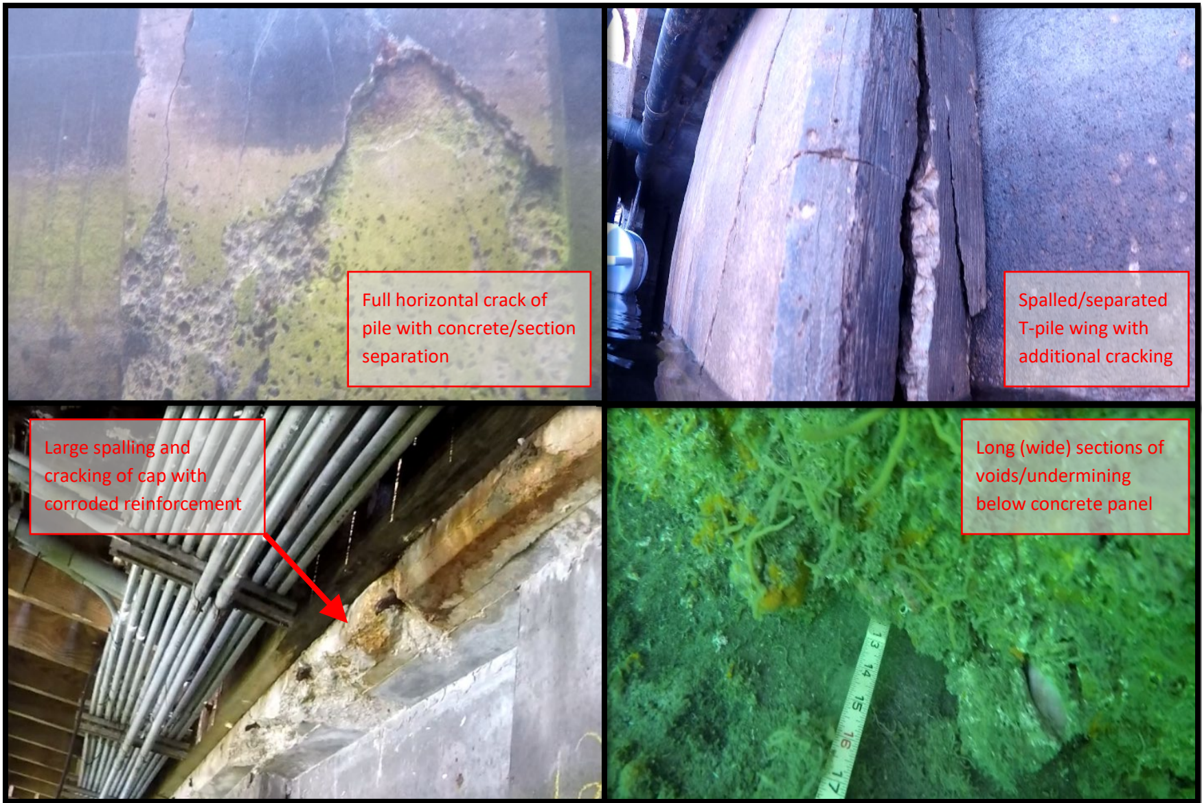
Figure 9: Typical Major Deficiencies – [Top Left] A-6 (Station 0+66), [Top Right] A-15 (Station 1+67), [Bottom Left] B-35 (Station 3+78), [Bottom Right] B-77 (Station 8+42 - 8+75)
