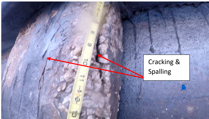
Deficiency A-21: Pile 30 (Station 2+26)
