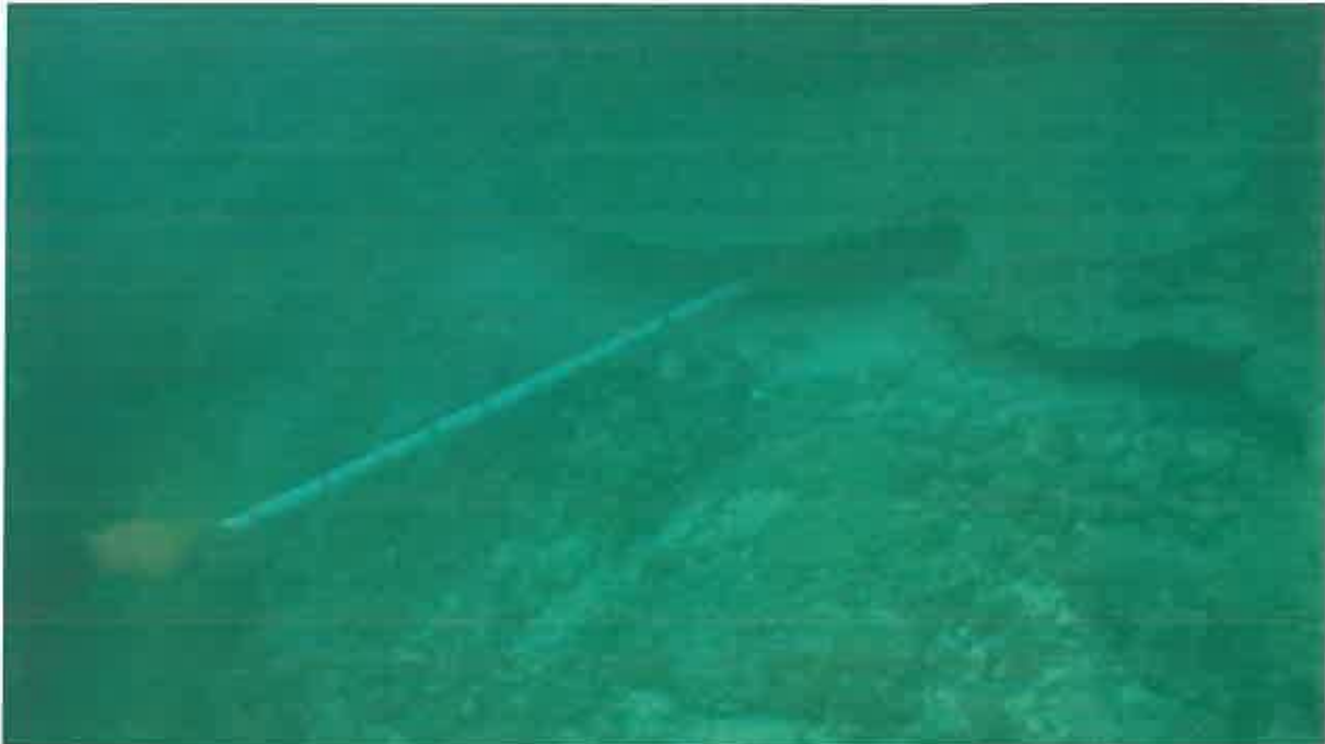
Undermining of the tremie concrete repairs at the base of the bulkhead. Note the steep slope of the dredge line.
