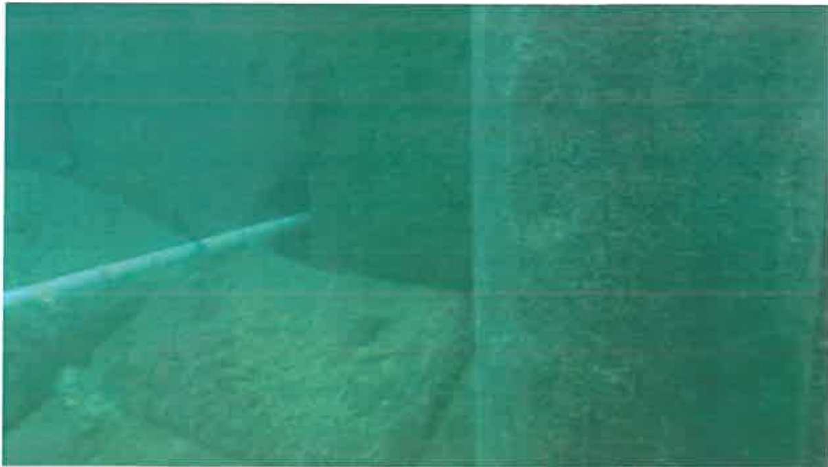
Quikrete concrete sacks placed in front of the sheet piling. Cavity evident above the sacks.
