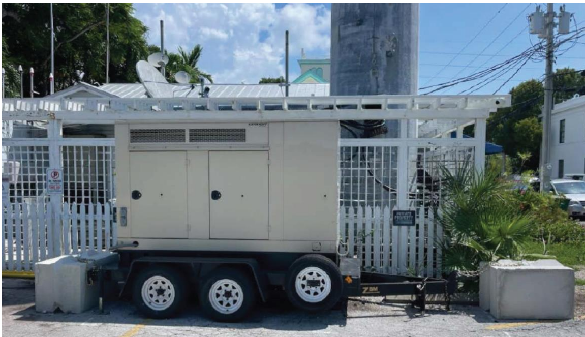
Photo of site under review with temporary generator to be removed.
