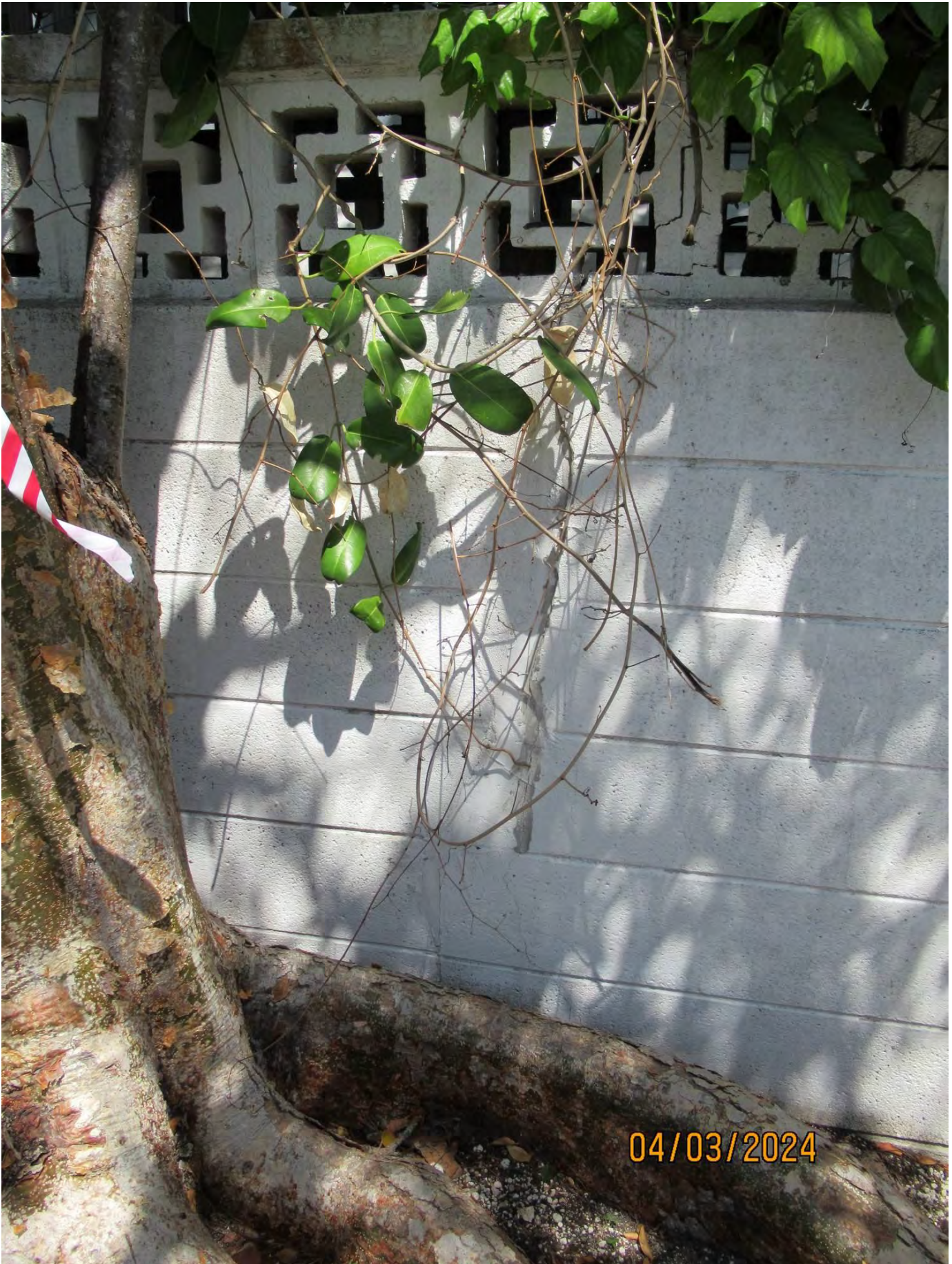
Photo showing cracks/damage to concrete property line wall I relation to the tree trunk and roots.
