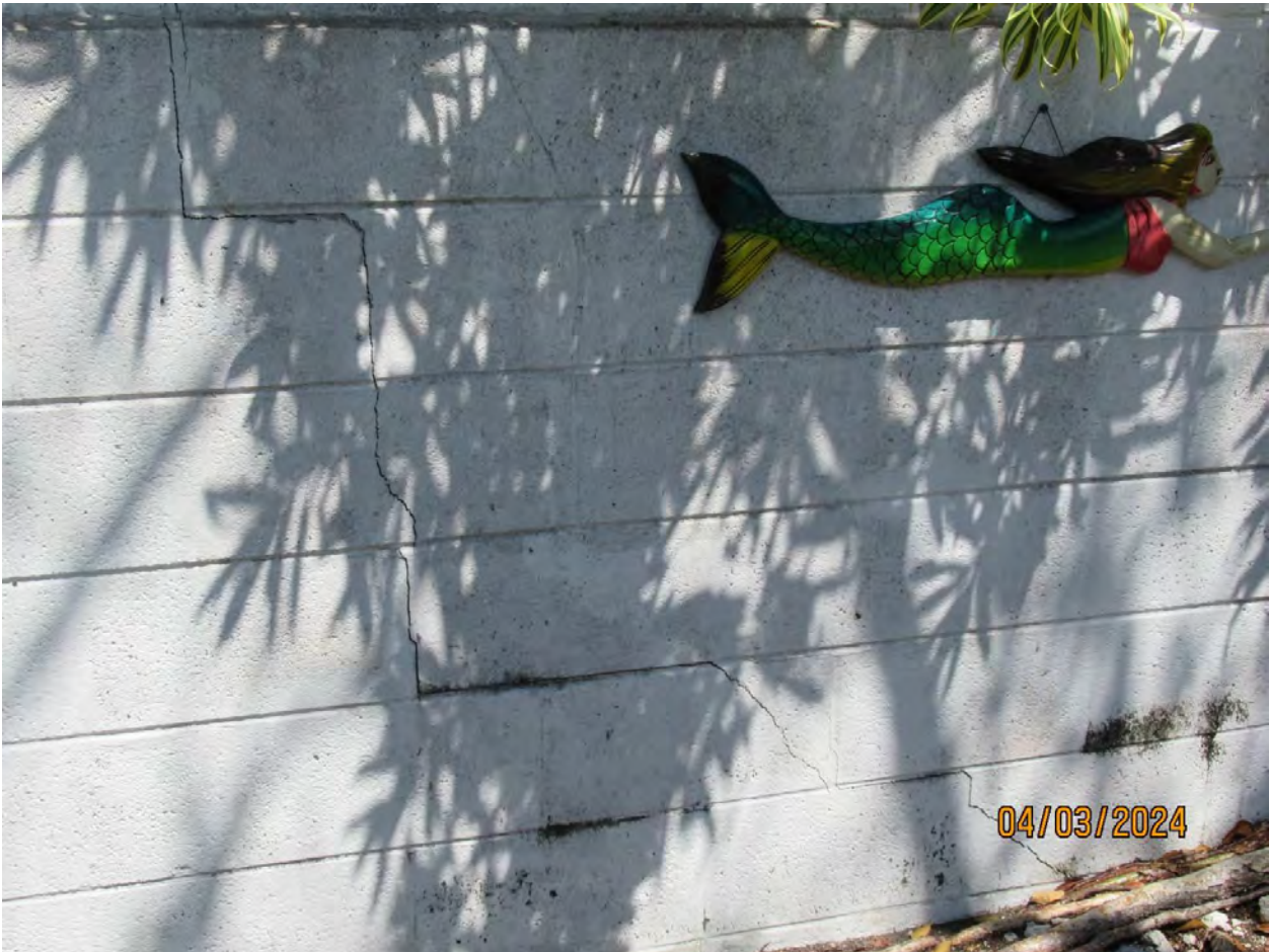
Photo of property line concrete wall showing cracks caused by tree/roots.
