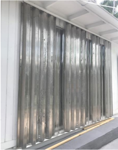
Metal/polycarbonate storm panels
