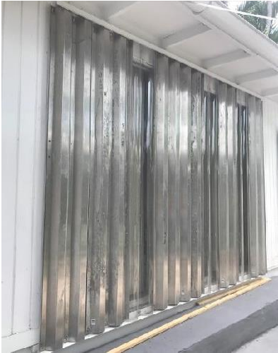
Metal/polycarbonate storm panels
