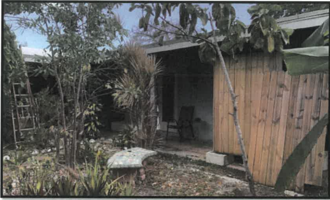
Lockout Unit attached to unit #9 - exterior
