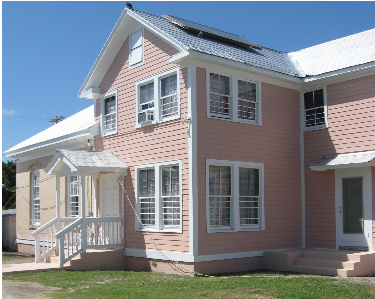
404 South Street before changing to 5 V-Crimp roofing. Notice the original masonry building to the left side.
