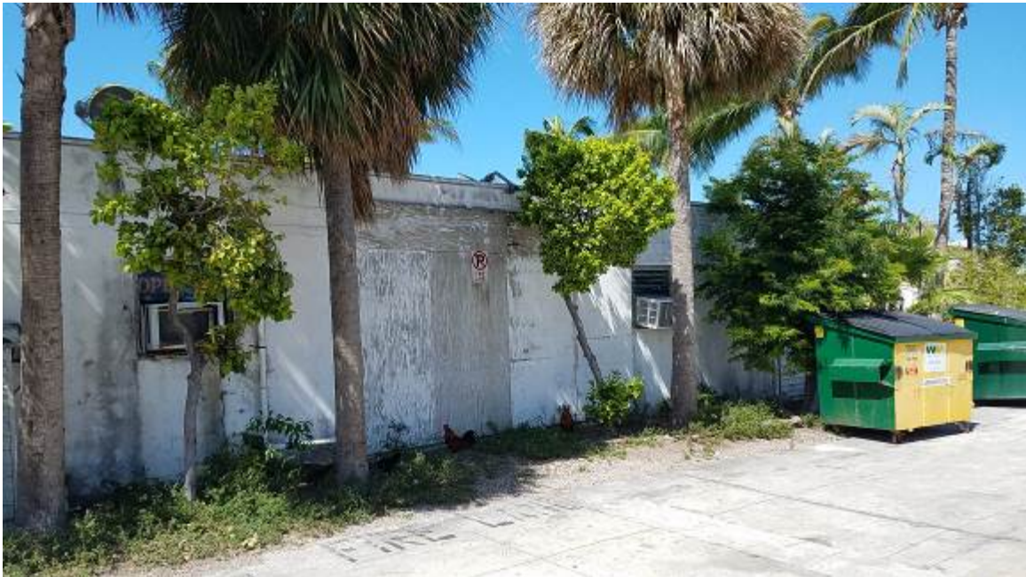
Figure 5. Partial right side elevation (middle of building). Large area covered with plywood which prevents damaged concrete debris from falling. Old paint and more damaged windows.
