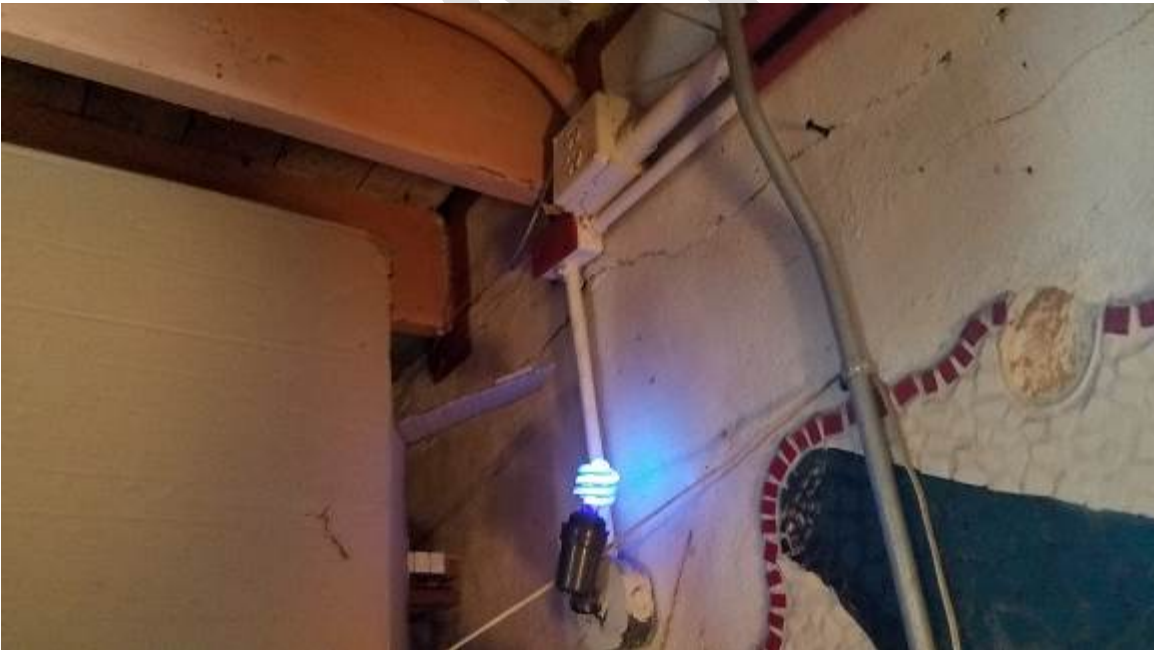
Figure 16. More electrical conduits, outlets and lights at the level of tie-beam and roof rafters requiring repairs.
