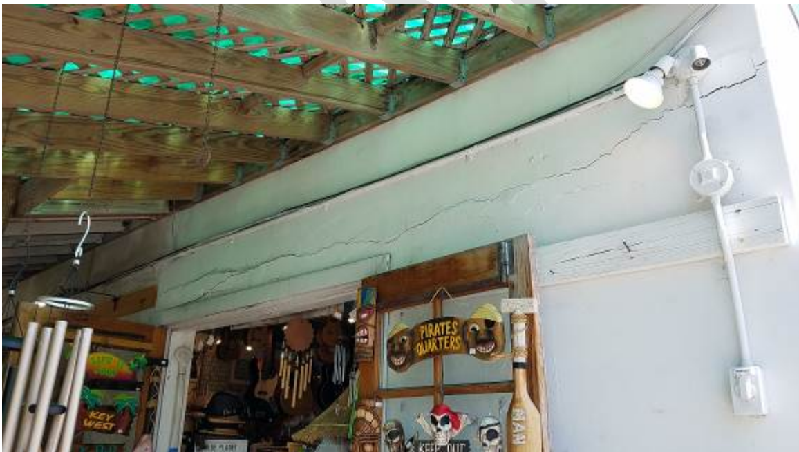
Figure 14. Heavy spalling damage above the side entrance into the gift shop. Large sections of concrete debris are unsecured and may fall creating life & health safety hazard. Roofing above with a patchwork of non-conforming improvements. More electrical components in the way of repairs.
