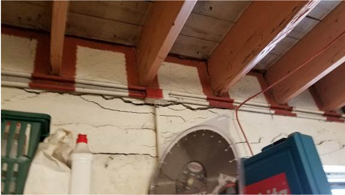
Figure 11. Same as above. Heavy concrete damage, damaged rafters and more electrical conduits.
