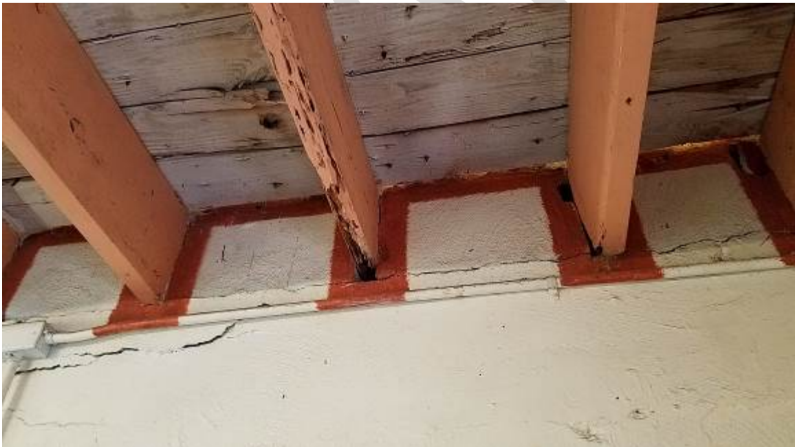
Figure 10. Maintenance shop - Interior view with damaged top of tie-beam and heavily damaged roof rafter. Damaged wood roofing deck. Please note electrical conduits along the tie-beam.
