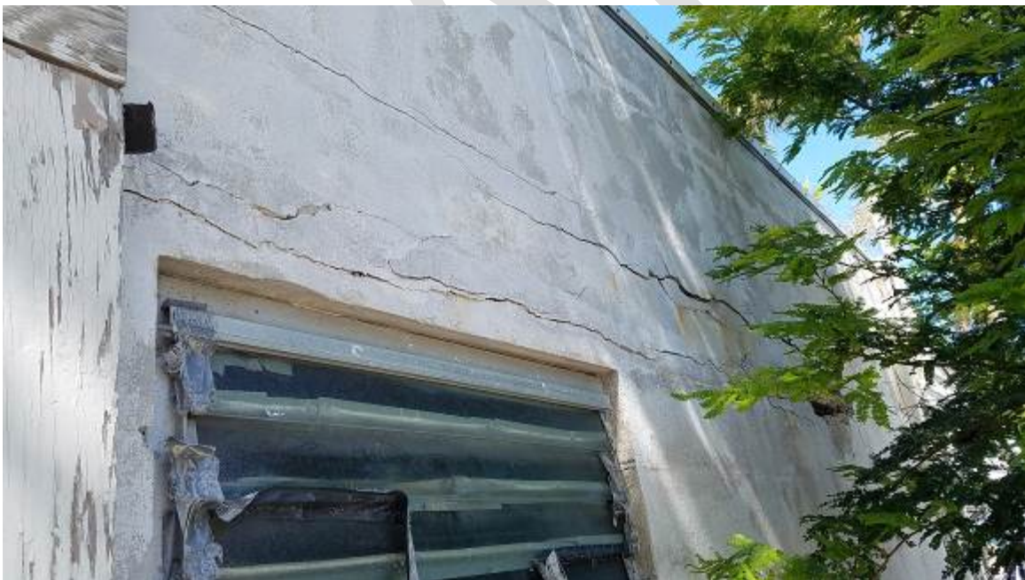
Figure 6. Same as above. Close-up view. Tie-beam with extensive damage and window sealed with duck tape.
