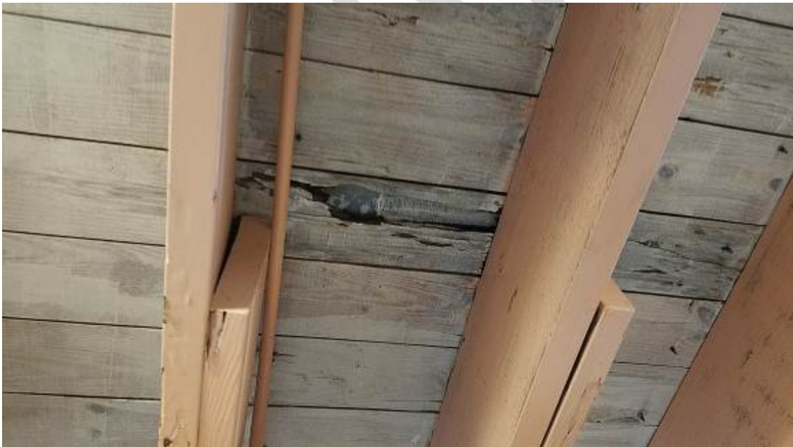
Figure 12. Roofing deck with hole demonstrating heavy termite damage to deck boards in some locations.
