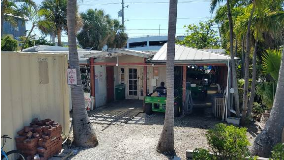
Figure 9. Rear elevation with pergola style and shed roof on the side. Rear of the shed is obstructed by storage container. Wood pergola and side roof are in poor shape but stable. Left side of the building is obstructed by the landscaping.
