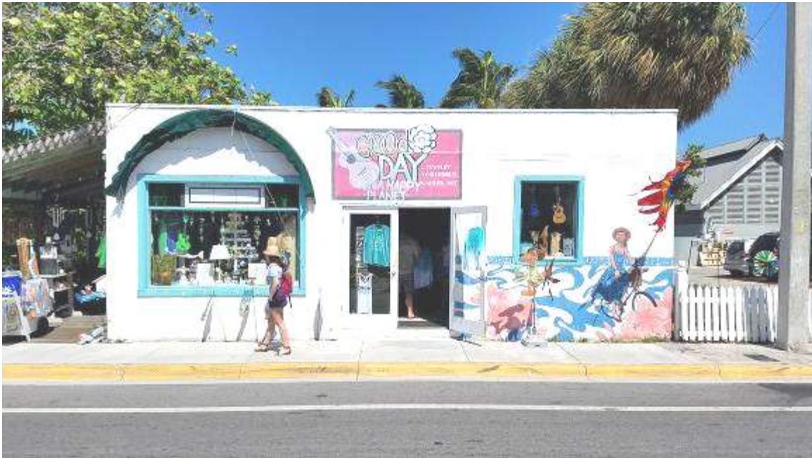
Figure 3. Front Elevation. Visible concrete damage – cracks along tie-beam above windows.
