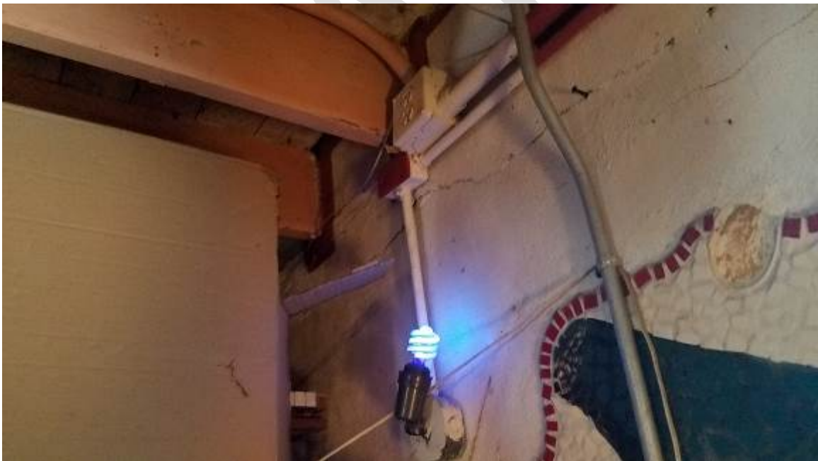
Figure 16. More electrical conduits, outlets and lights at the level of tie-beam and roof rafters requiring repairs.
