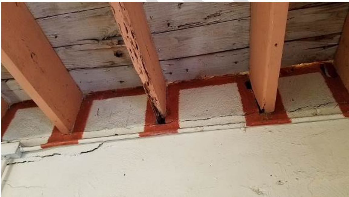
Figure 10. Maintenance shop - Interior view with damaged top of tie-beam and heavily damaged roof rafter. Damaged wood roofing deck. Please note electrical conduits along the tie-beam.
