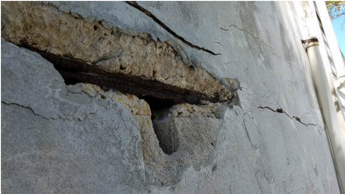
Figure 7. Same as above. Rear of the building right side. Large parts of the tie-beam collapsed, and damaged reinforcement exposed to the elements.
