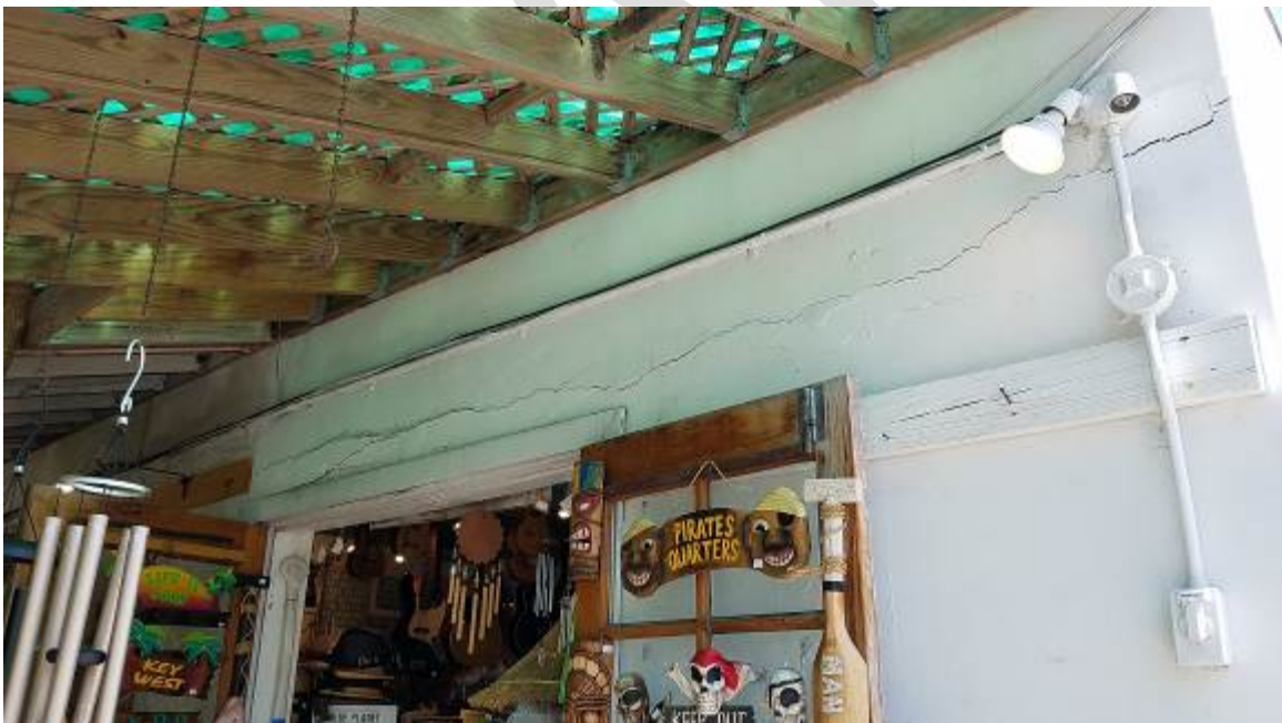
Figure 14. Heavy spalling damage above the side entrance into the gift shop. Large sections of concrete debris are unsecured and may fall creating life & health safety hazard. Roofing above with a patchwork of non-conforming improvements. More electrical components in the way of repairs.
