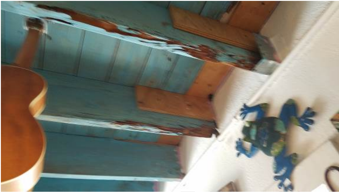
Figure 15. Heavy termite damage to the rafters (interior of the gift shop).
