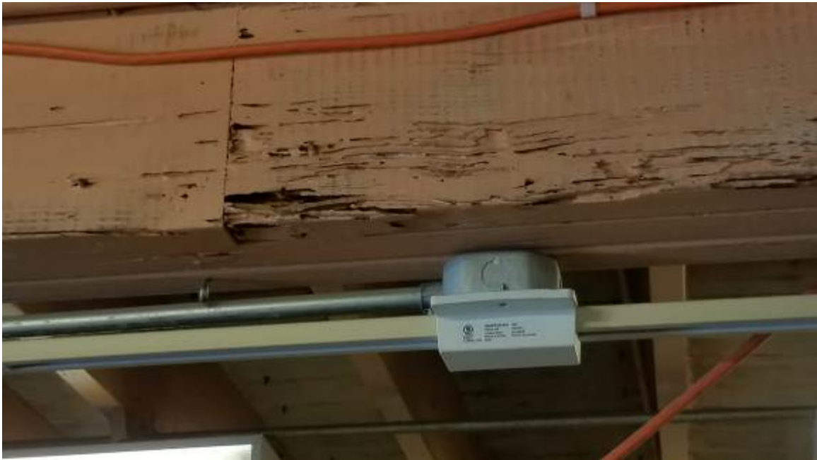
Figure 13. Termite damage to the middle roof beam and attached electrical components.
