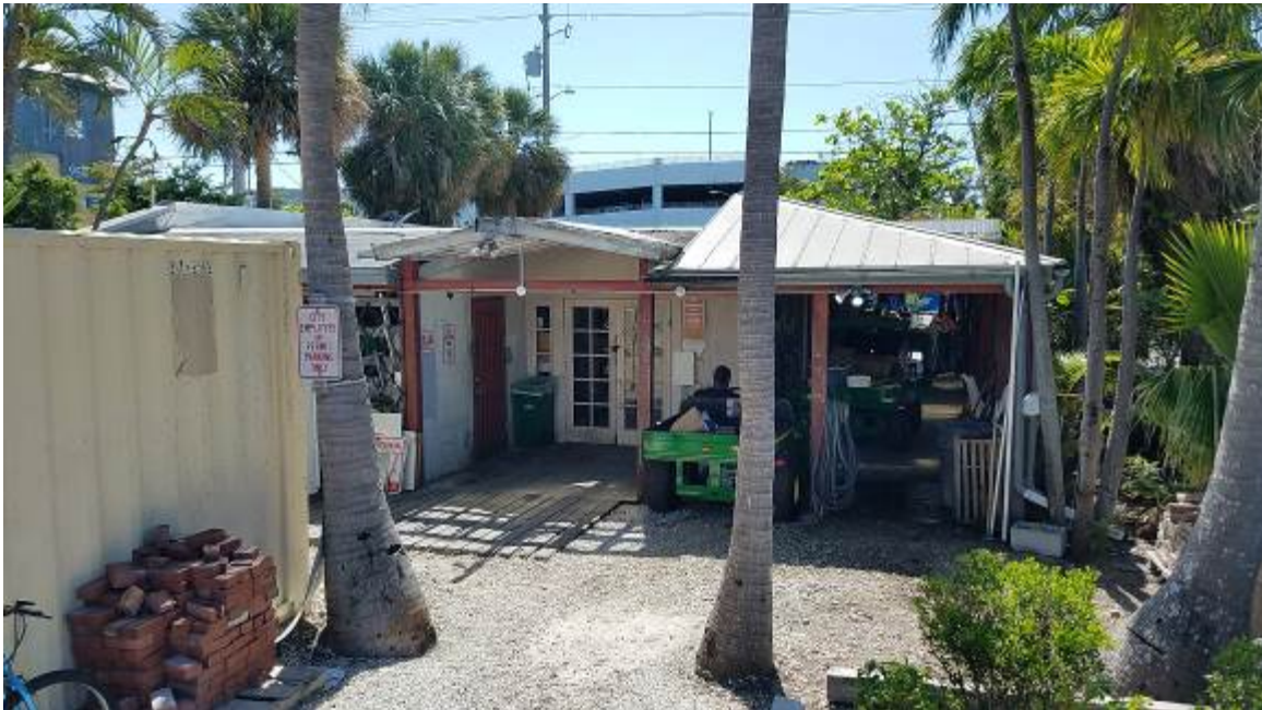
Figure 9. Rear elevation with pergola style and shed roof on the side. Rear of the shed is obstructed by storage container. Wood pergola and side roof are in poor shape but stable. Left side of the building is obstructed by the landscaping.
